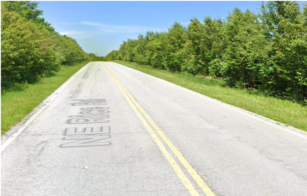
Lack of Acceleration and Deceleration Lanes
