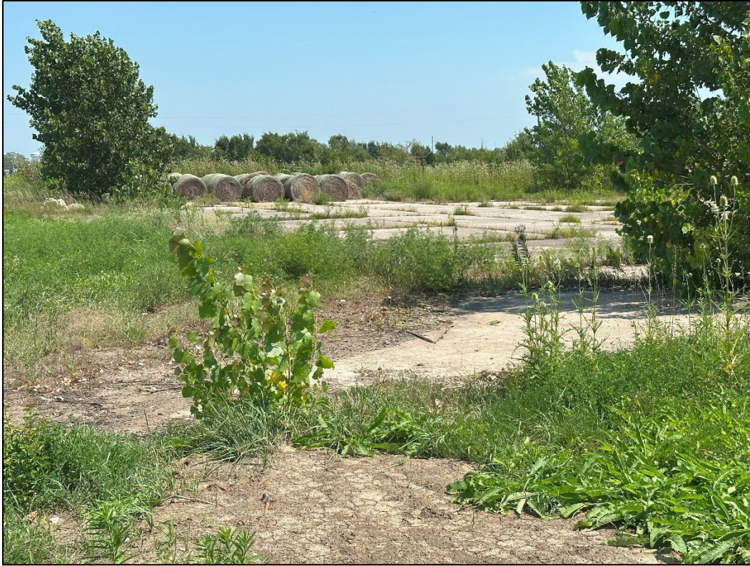
1001 S. M-291 – looking east – deterioration of pavement; overgrown vegetation
