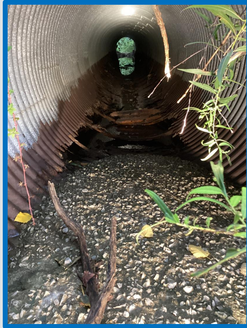
Bottom portion of pipe is completely missing.
