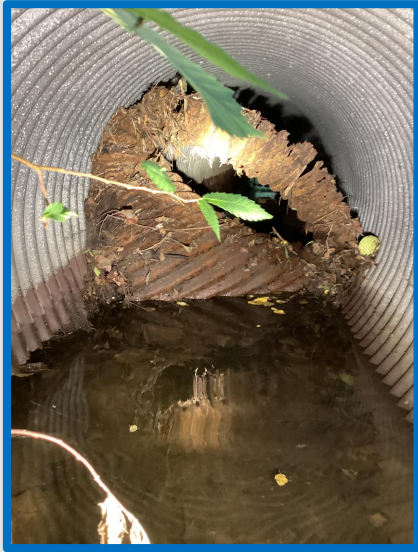
Along this run of pipe, the bottom portion was displaced and rolled up blocking much of the pipe.
