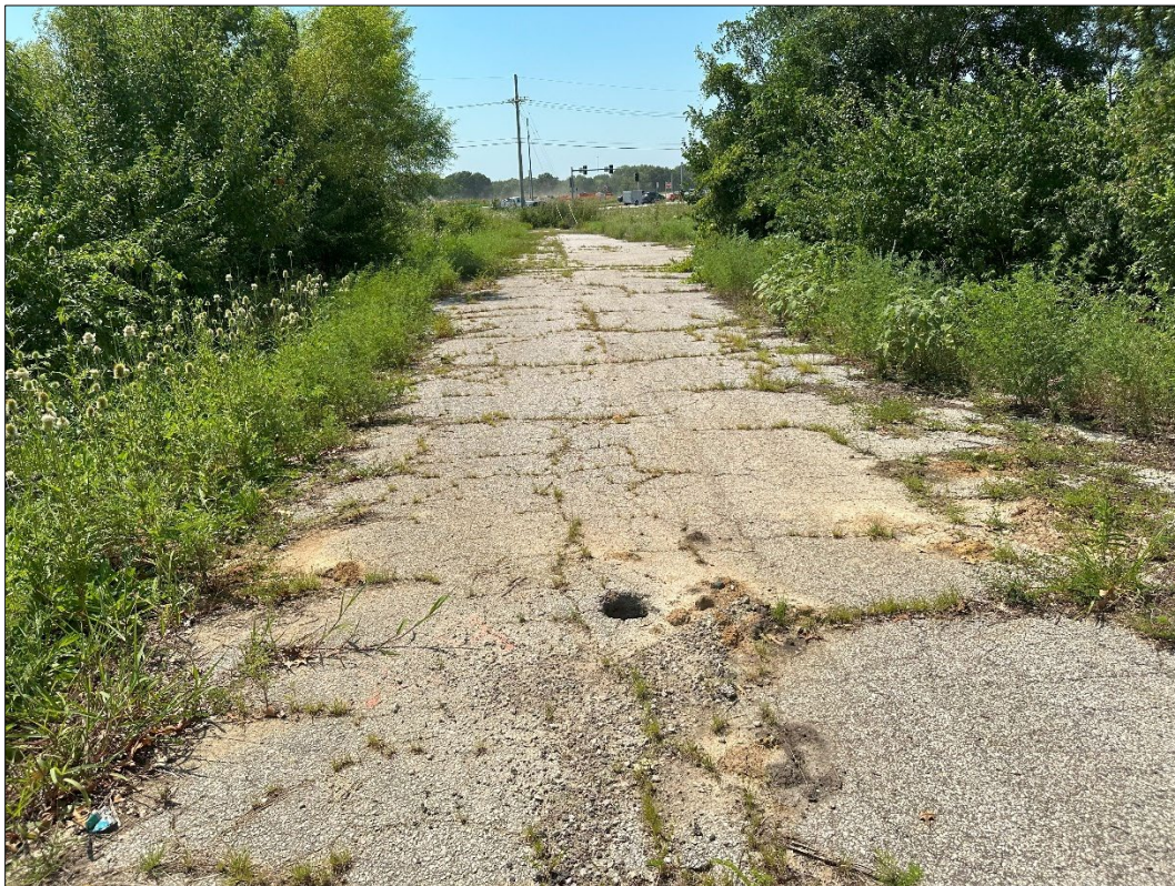
1001 S. M-291 – looking west – deterioration of pavement; overgrown vegetation
