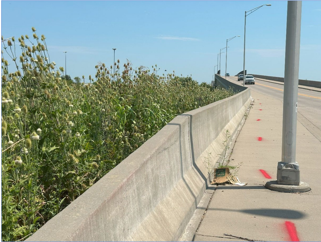
1 Pfizer Way – looking east along SE Bailey Rd – overgrown vegetation
