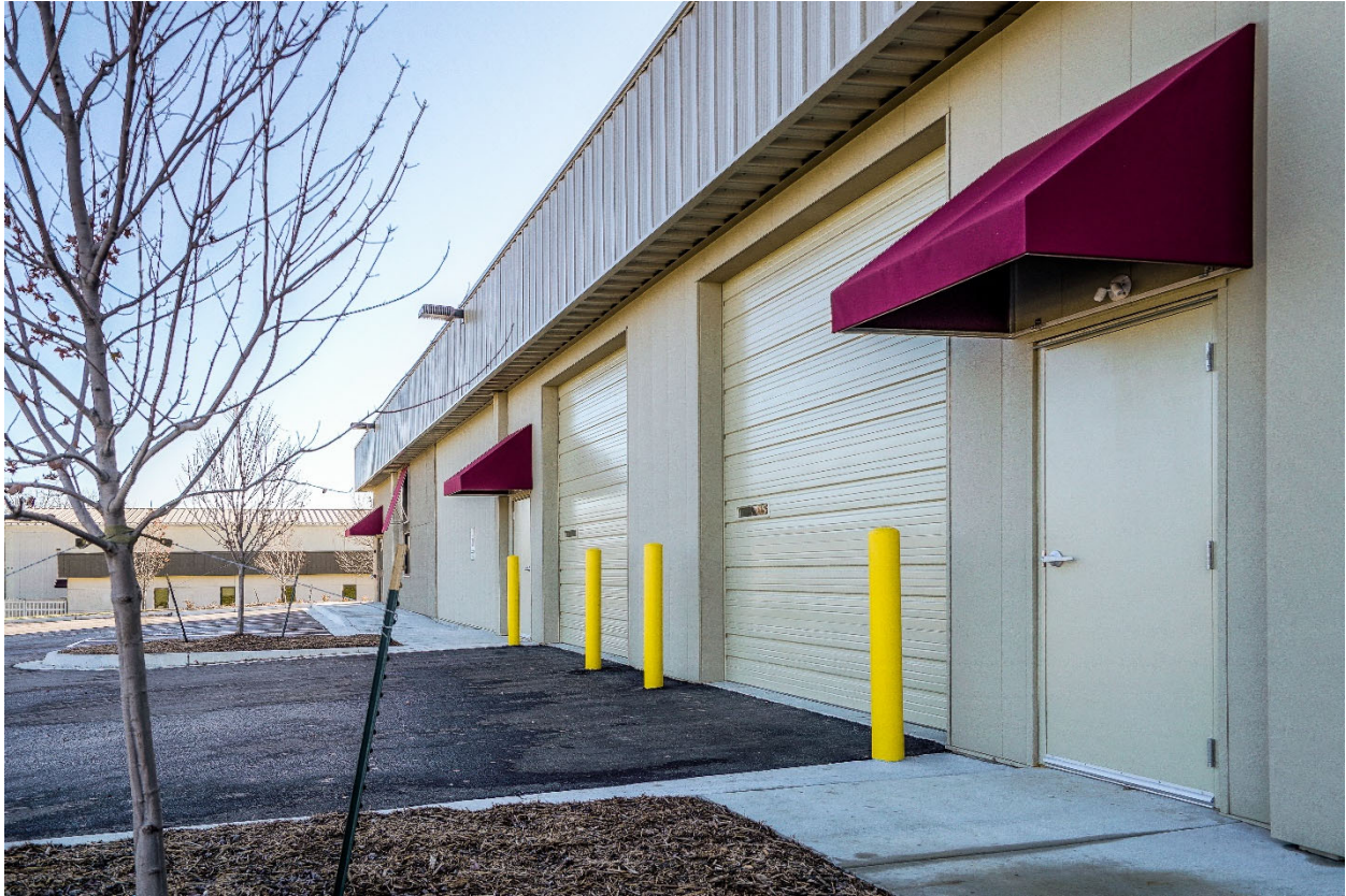
Textured Stucco finish flat metal wall panel used at Shamrock Business Park
