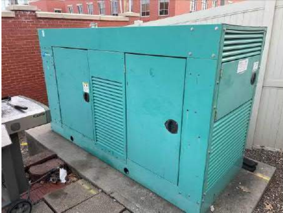
Photo #13 View of natural gas emergency generator
