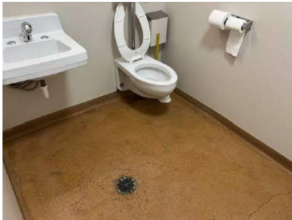
Photo #9 Typical on-site bathroom with floor drain
