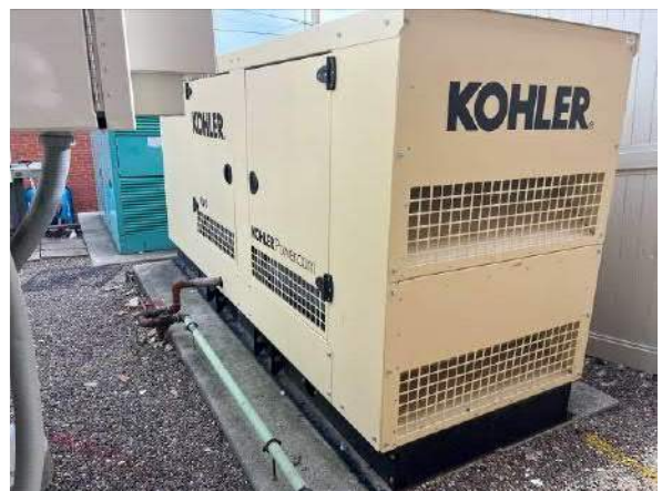
Photo #12 View of natural gas emergency generator
