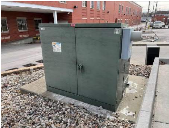
Photo #15 View of on-site pad-mounted transformer
