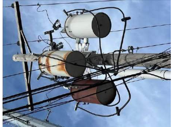
Photo #14 View of on-site pole-mounted transformers
