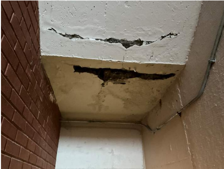
Figure 1: North exit stair concrete spall.
