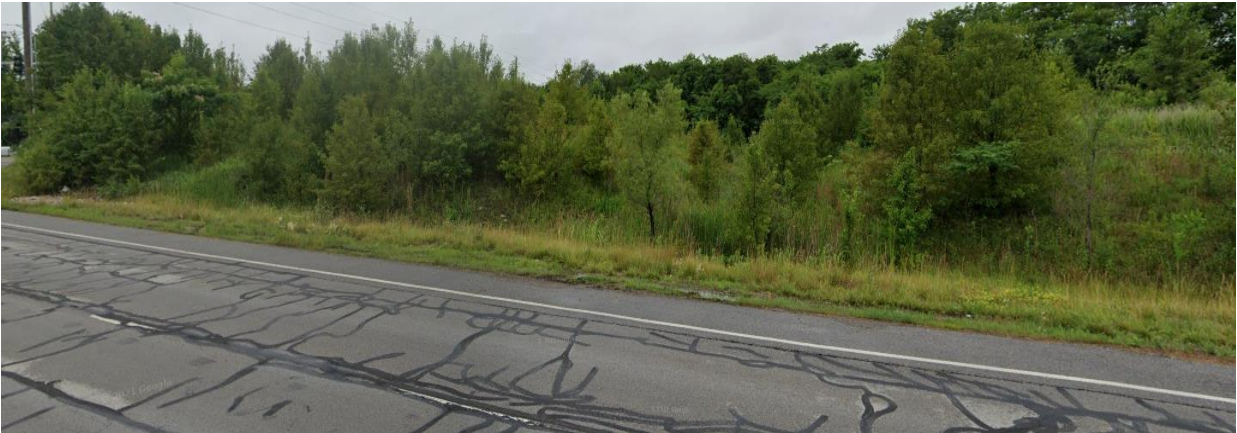
Overgrown Vegetation Along NE Todd George Parkway
