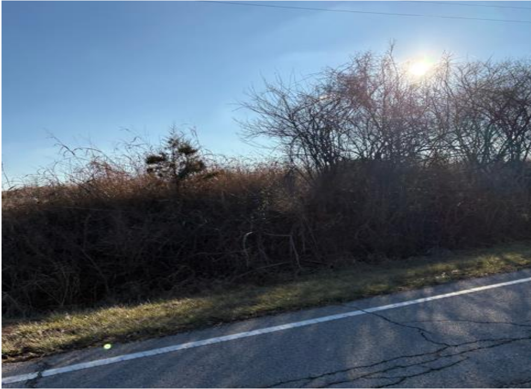
Overgrown Vegetation Along Public Road
