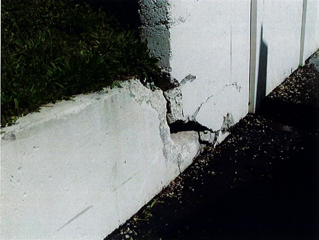
Photo 15 – Deteriorated/compromised retaining wall.
