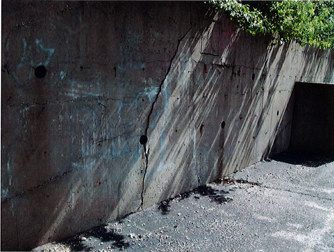
Photo 10 – Deteriorated/compromised retaining wall.
