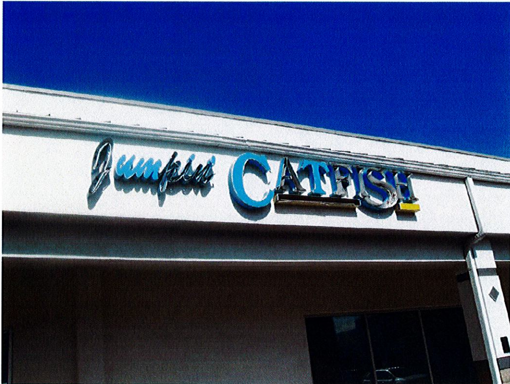
Photo 4 – Deteriorated/damaged tenant signage.
