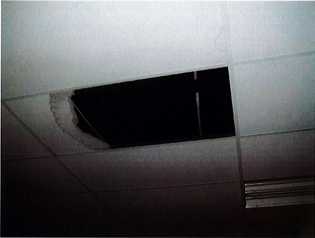
Photo 29 – Interior ceiling tile deterioration.
