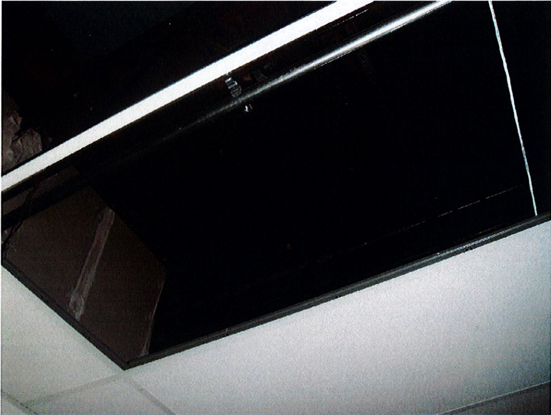
Photo 33 – Roof structure condensation.
