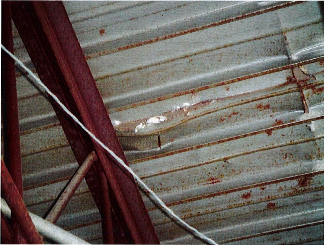
Photo 25 – Roof structure deterioration.
