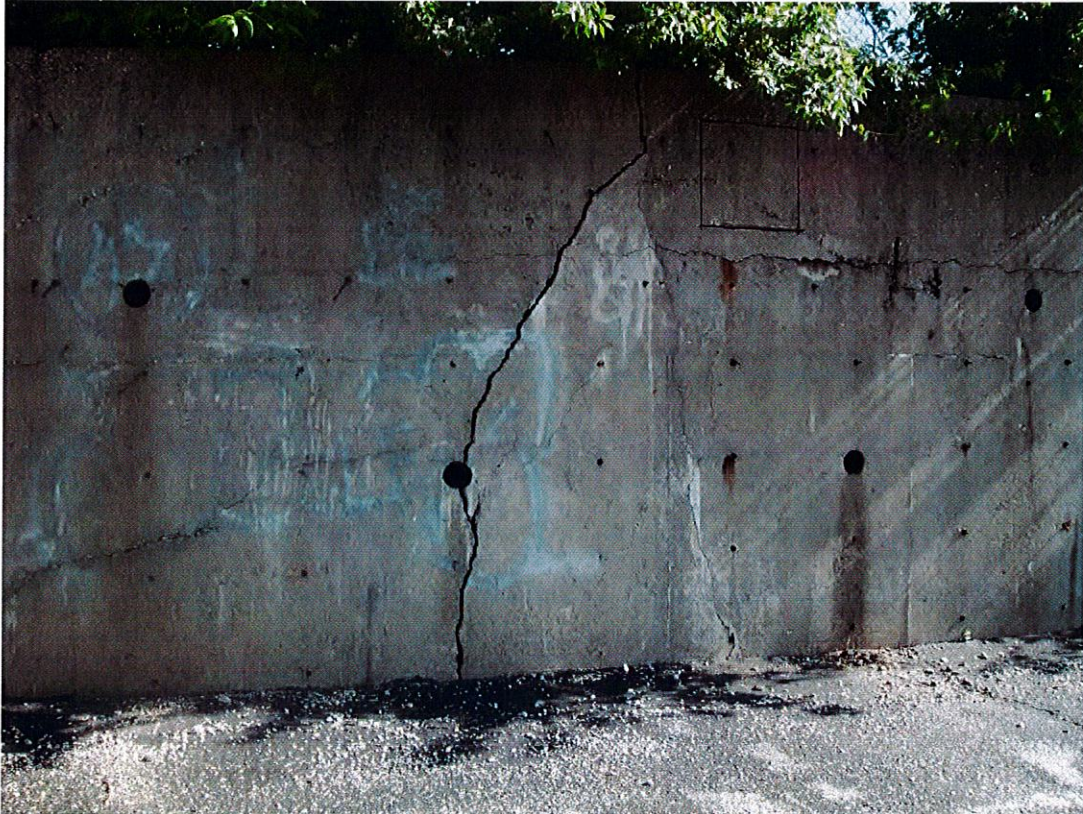
Photo 7 – Graffiti along west and north retaining wall.
