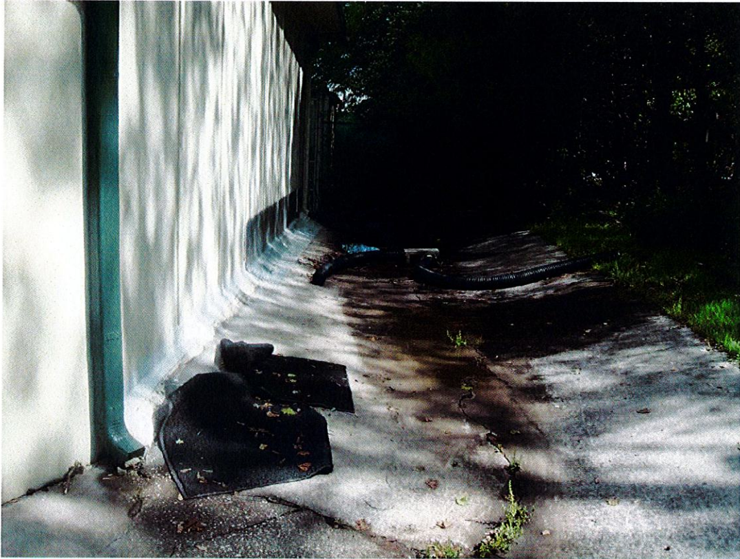
Photo 41 – Inadequate drainage area.
