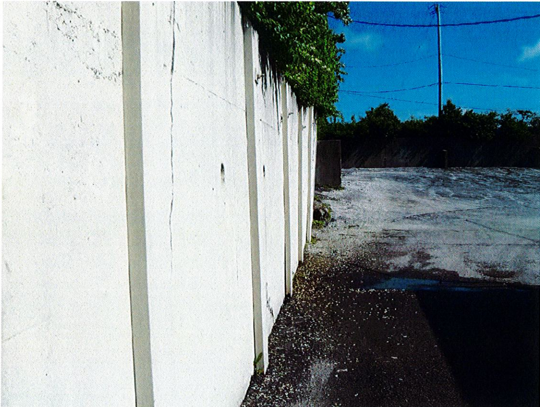
Photo 16 – Deteriorated/compromised retaining wall.
