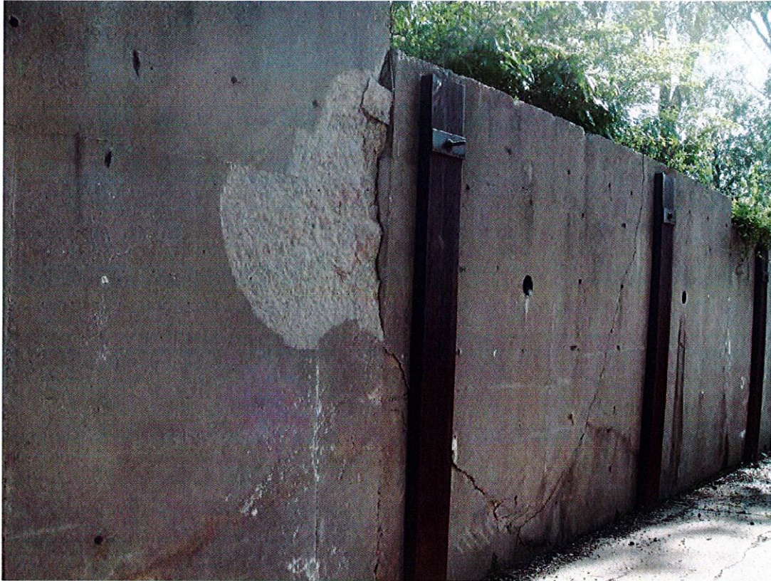
Photo 9 – Deteriorated/compromised retaining wall.
