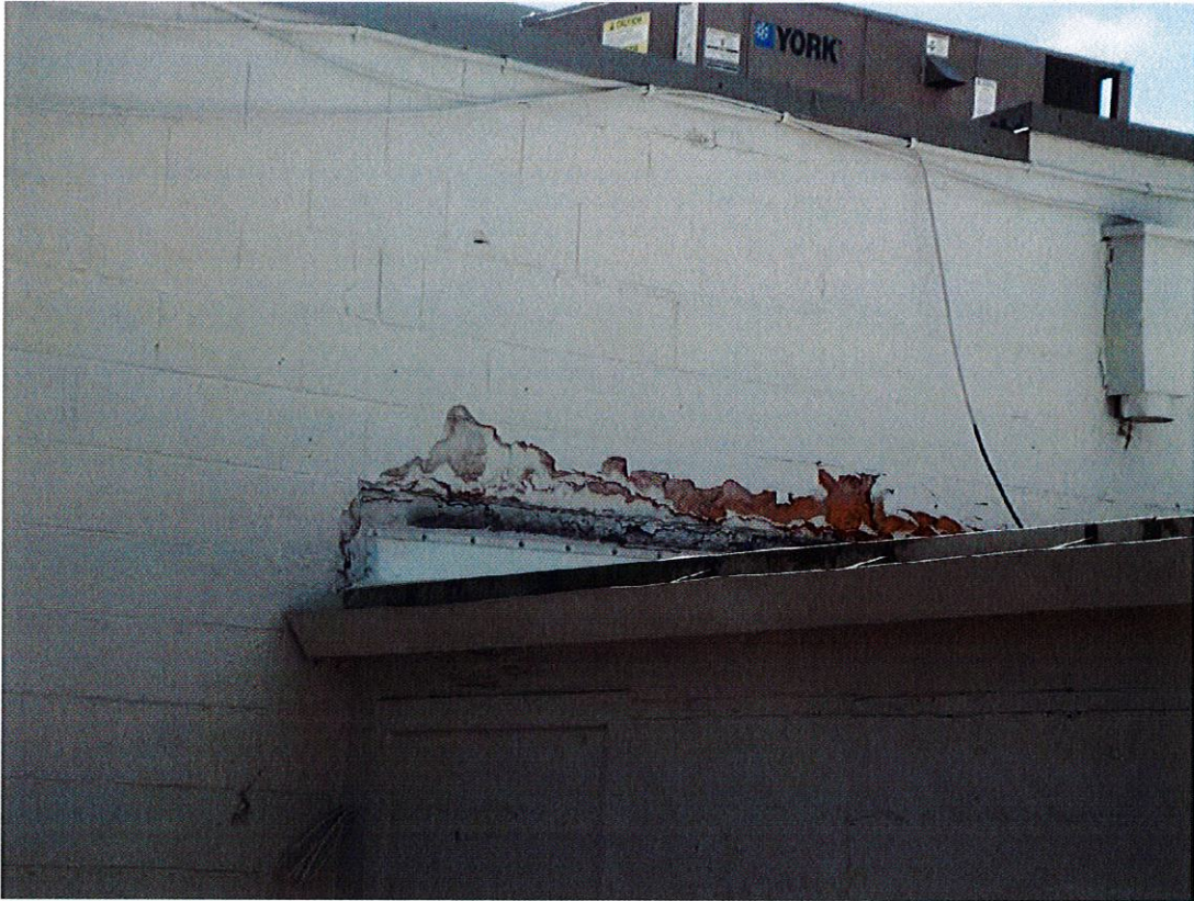
Photo 21 – Deteriorated flashing material.
