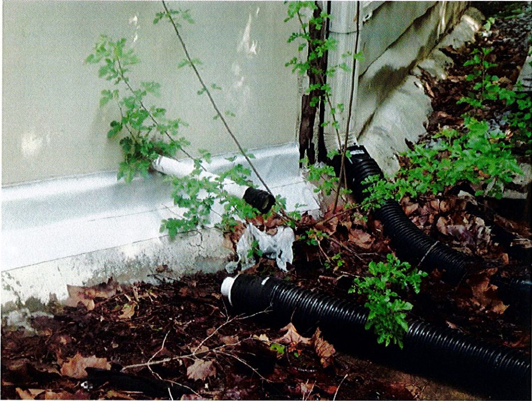
Photo 45 – Inadequate drainage area.
