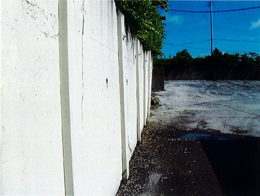
Photo 16 – Deteriorated/compromised retaining wall.
