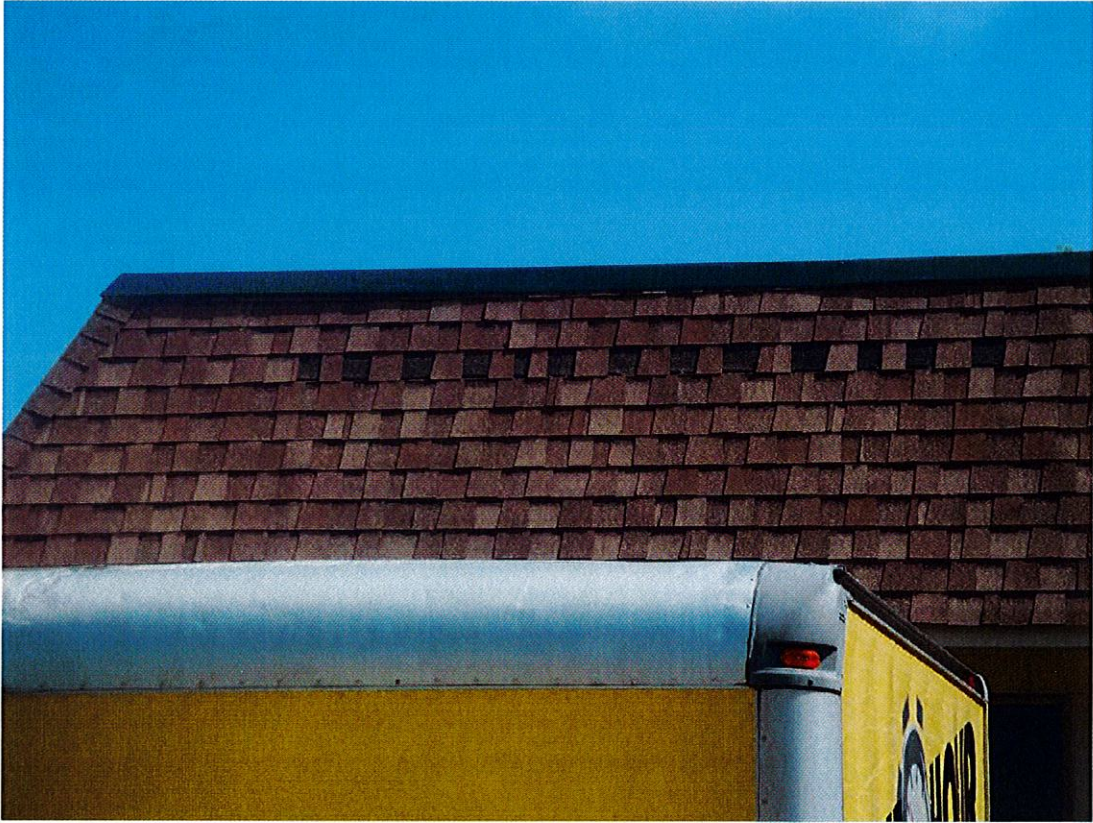
Photo 46 – Deteriorating roofing material.
