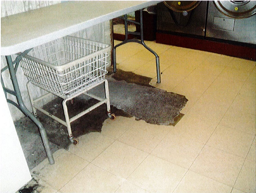
Photo 36 – Deteriorated/damaged floor tile.
