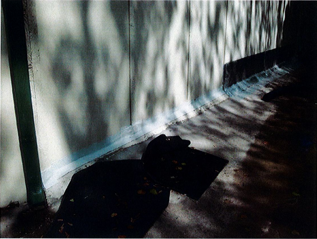
Photo 43 – Inadequate drainage area.
