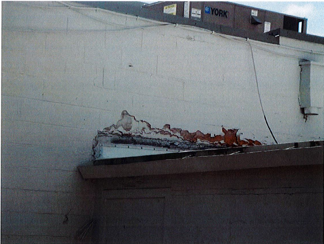
Photo 21 – Deteriorated flashing material.
