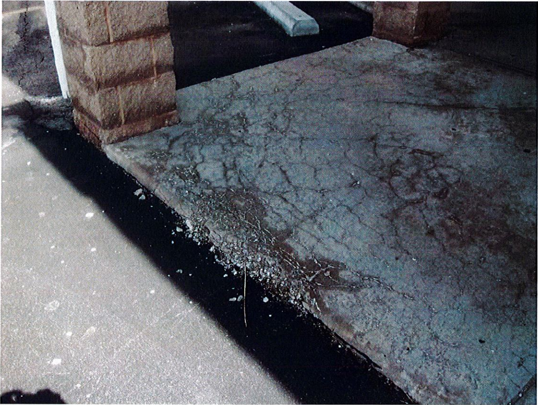
Photo 18 – Deteriorating concrete sidewalk.
