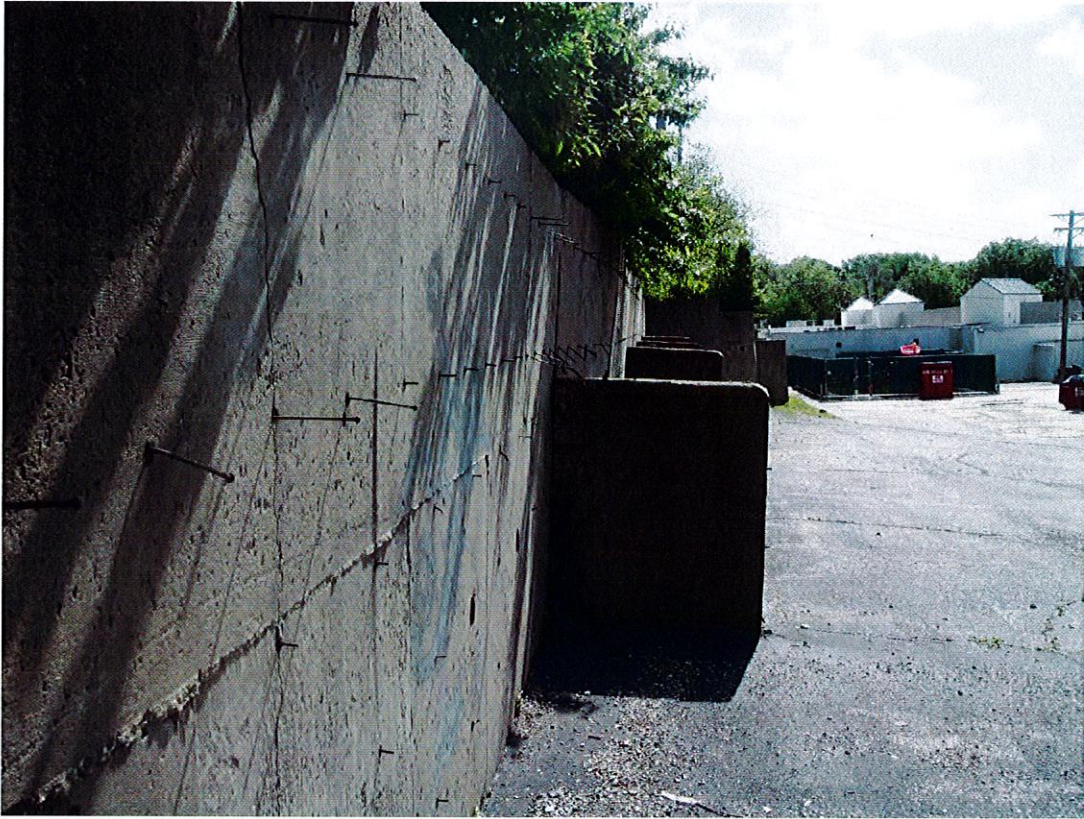
Photo 11 – Deteriorated/compromised retaining wall.
