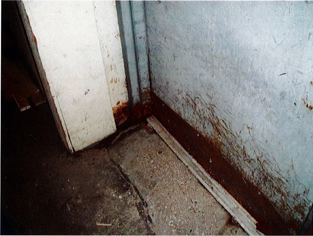
Photo 35 – Deteriorating exterior tenant door.
