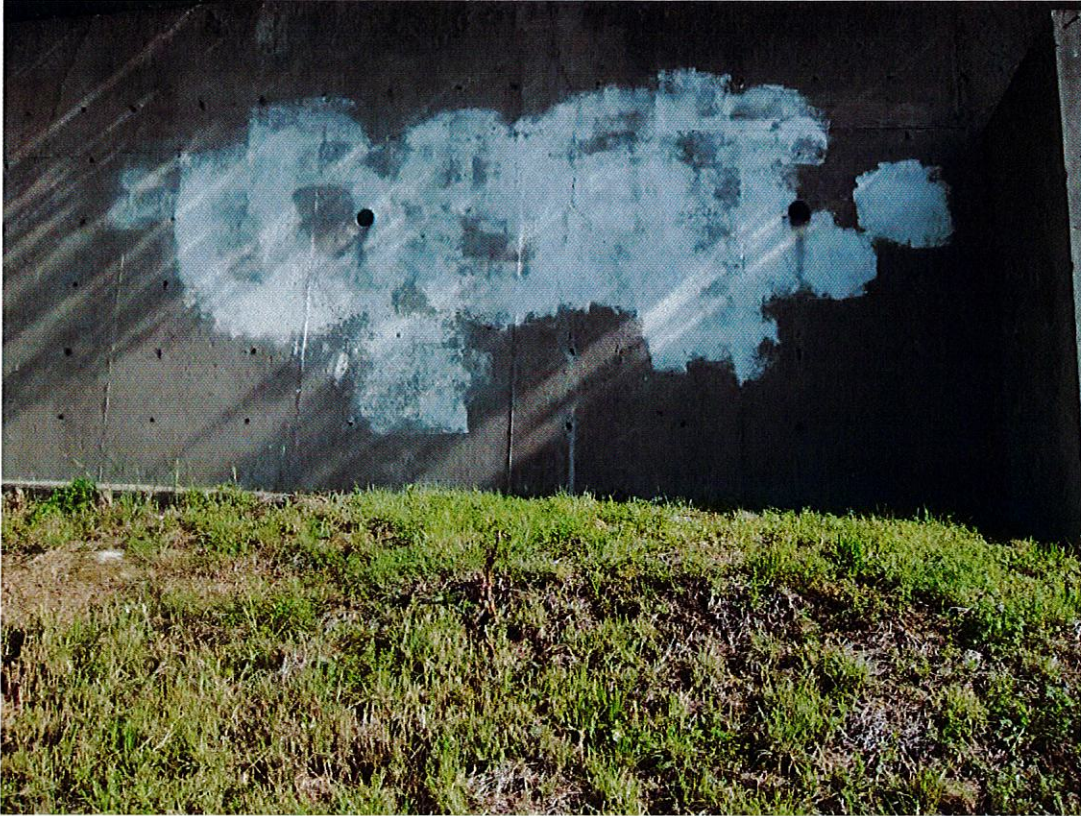
Photo 8 – Graffiti along west and north retaining wall.
