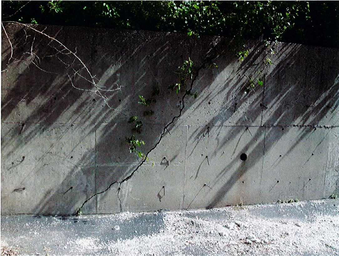
Photo 12 – Deteriorated/compromised retaining wall.
