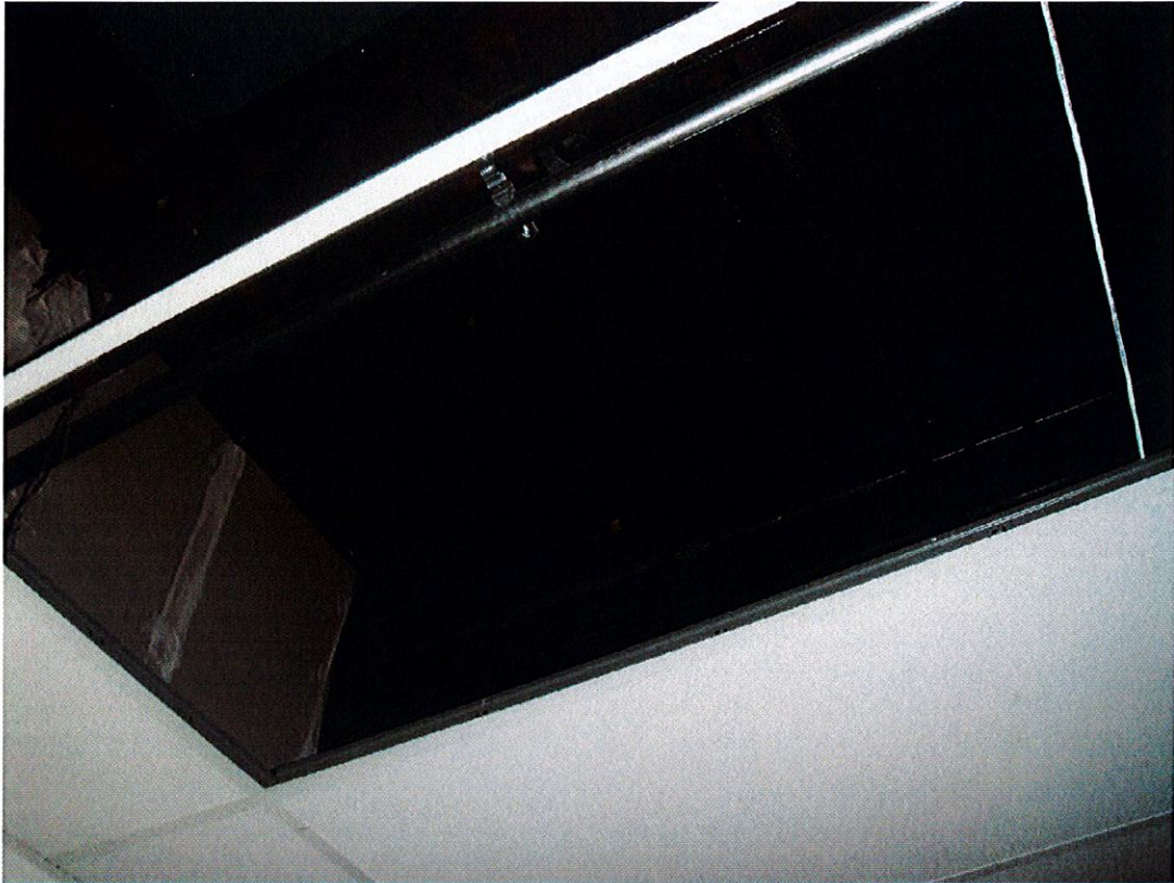
Photo 33 – Roof structure condensation.
