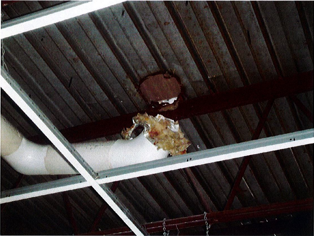
Photo 26 – Roof structure deterioration.
