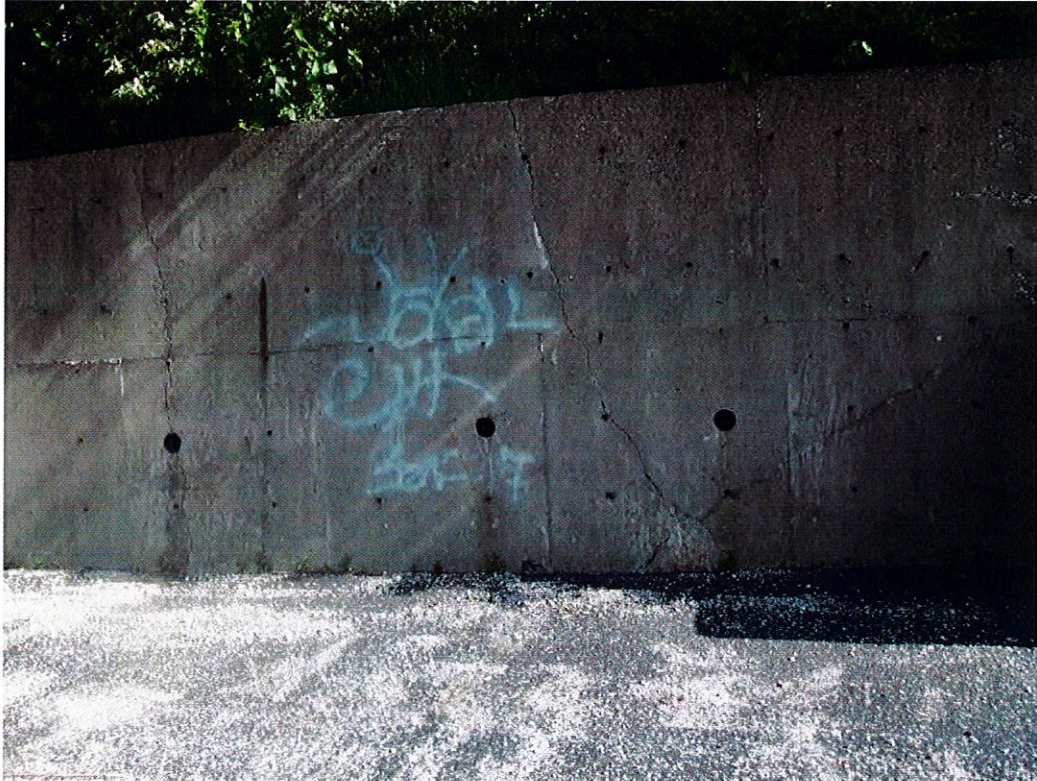
Photo 6 – Graffiti along west and north retaining wall.
