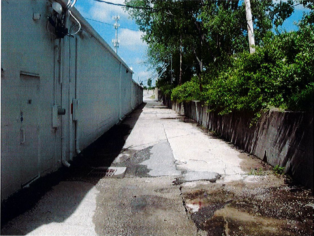
Photo 22 – View of north service alley. Typical of alley condition. Photo looking west.
