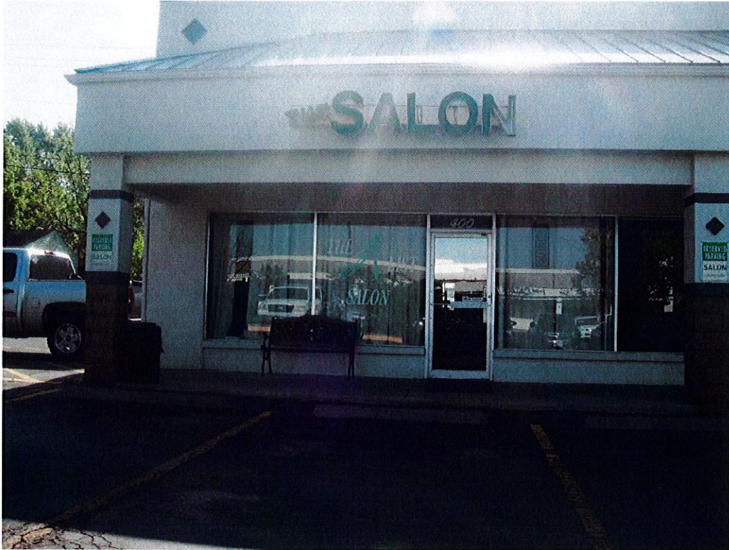
Photo 5 – Deteriorated/damaged tenant signage.
