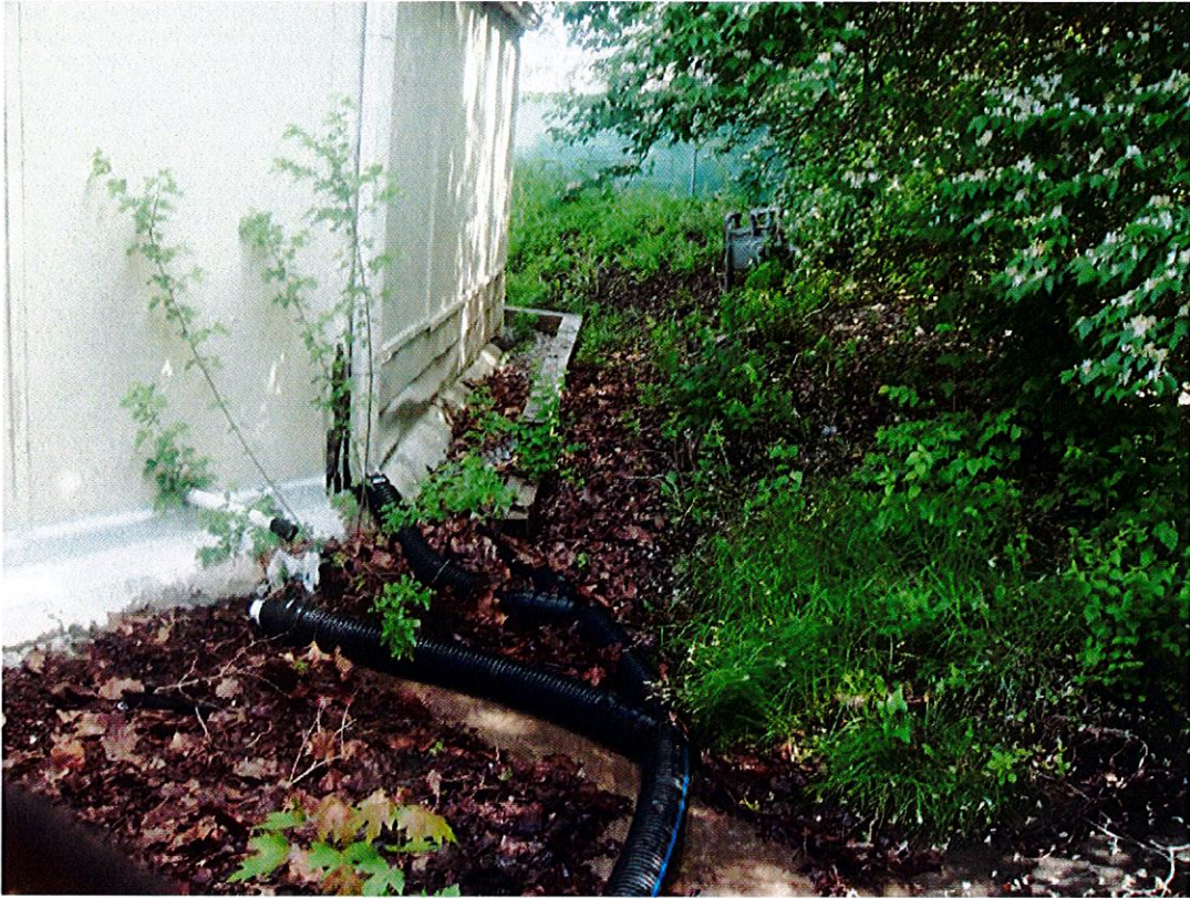
Photo 44 – Inadequate drainage area.
