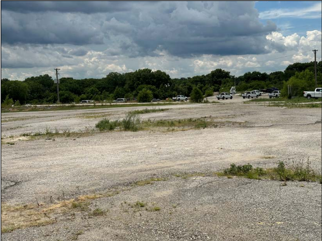
101 SW Oldham Pkwy – deterioration of pavement; overgrown vegetation
