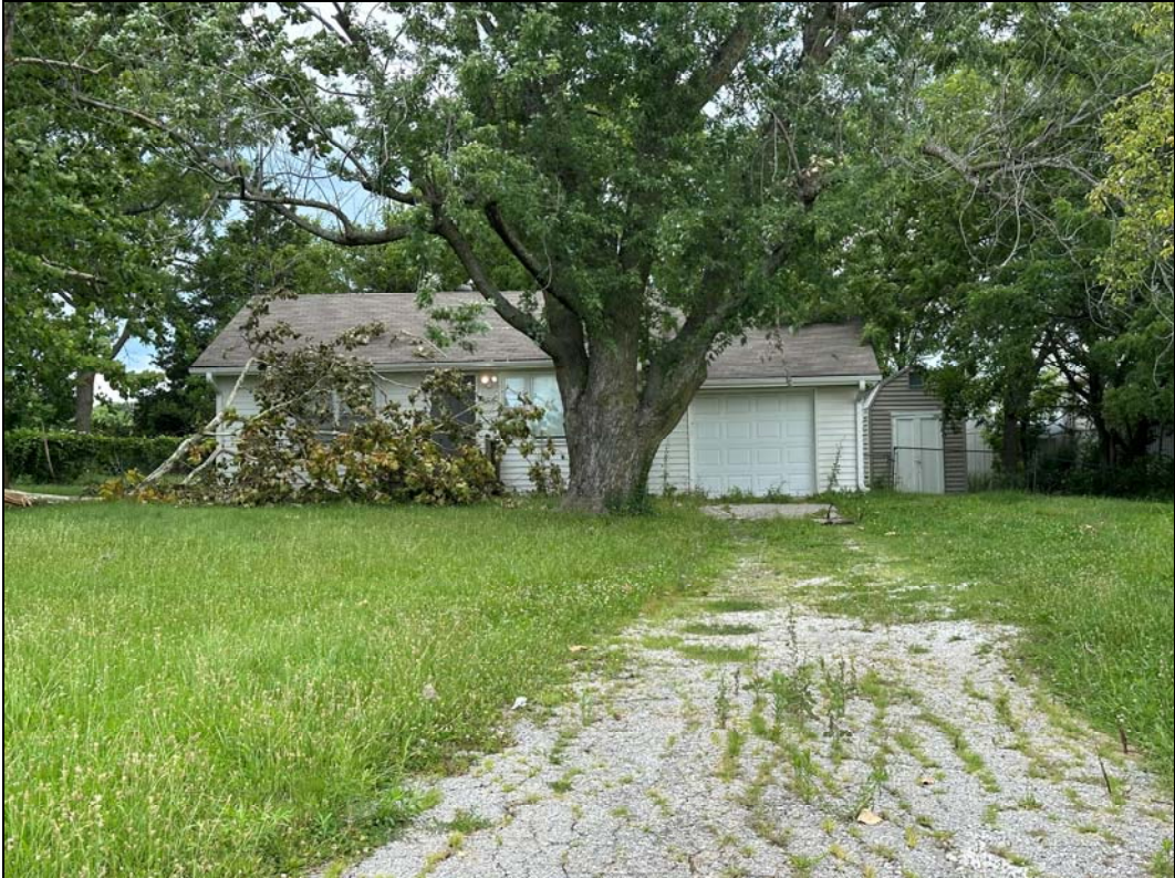
1208 SW Jefferson St – deterioration of driveway; vegetative debris
