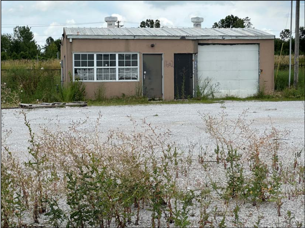
1206 SW Market St – deterioration of roof, fascia, gutter and downspouts, doors, and failure of finishes
