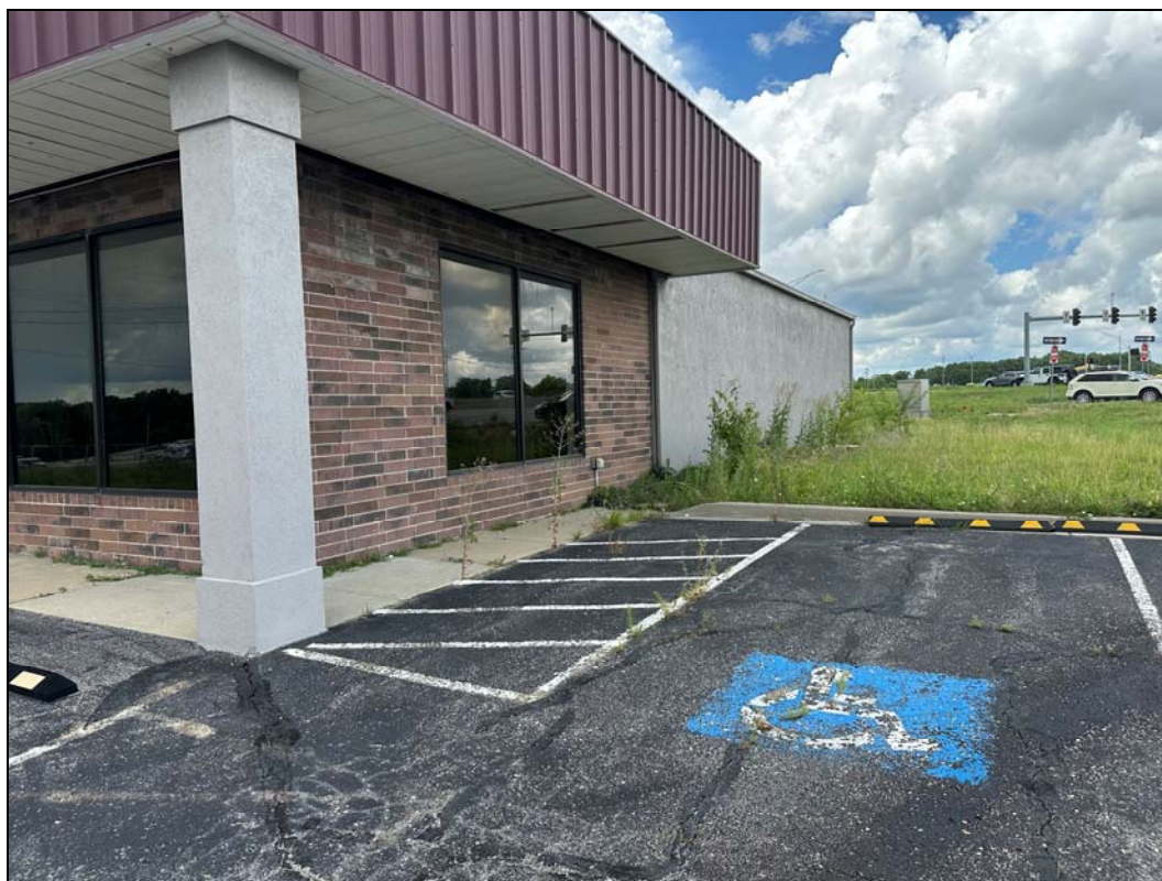
1025 SW Jefferson St – noncompliance with ADA (signage); overgrown vegetation
