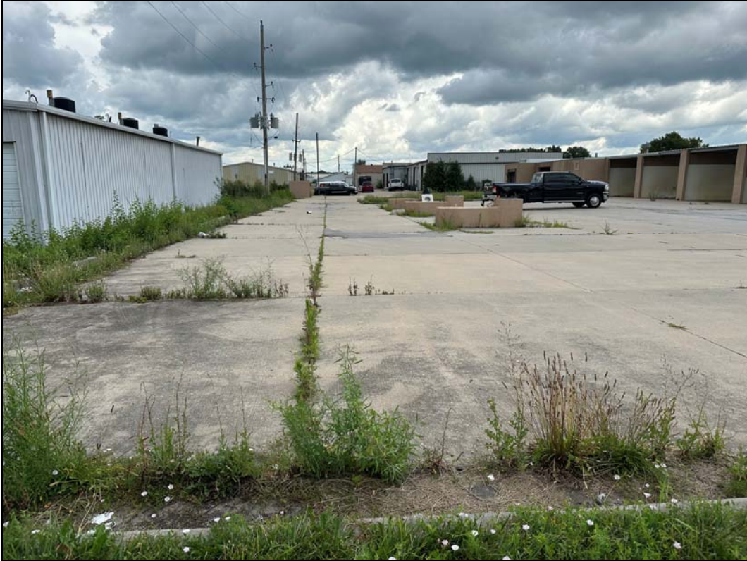
1310 SW Market St – overgrown vegetation; trash/debris; deterioration of pavement
