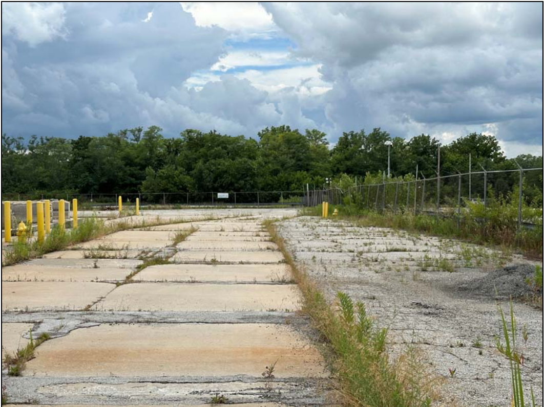
1204 SW Jefferson St – deterioration of pavement, fence; overgrown vegetation
