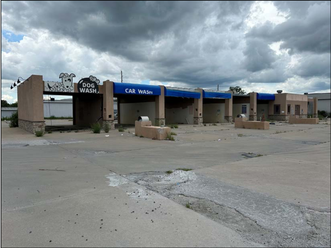
3049 William St – deterioration of parking pavement
