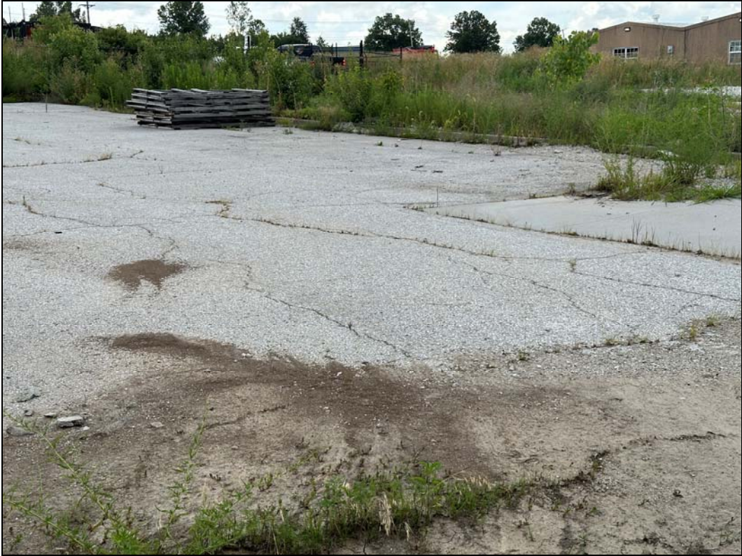
1051 SW Jefferson St – deterioration of parking lot; trash/debris; overgrown vegetation
