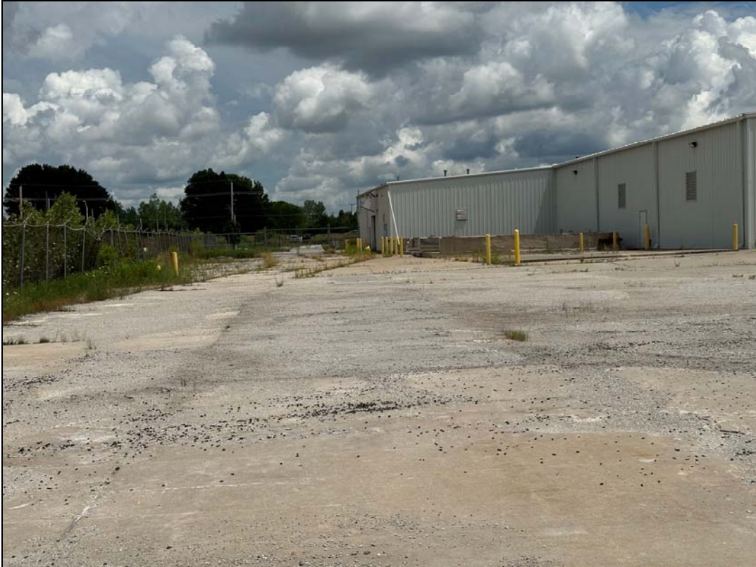
1204 SW Jefferson St – deterioration of pavement, fence; overgrown vegetation; failure of finishes
