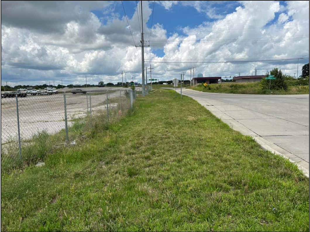
101 SW Oldham Pkwy – non-existent pedestrian circulation; deterioration of pavement
