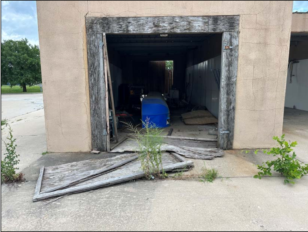
1310 SW Market St – deterioration of doors; open building; cracks in EIFS/stucco
