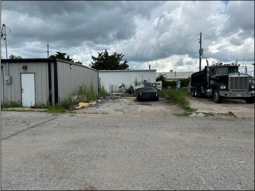
1301 SW Jefferson St – deterioration of drive aisle pavement
