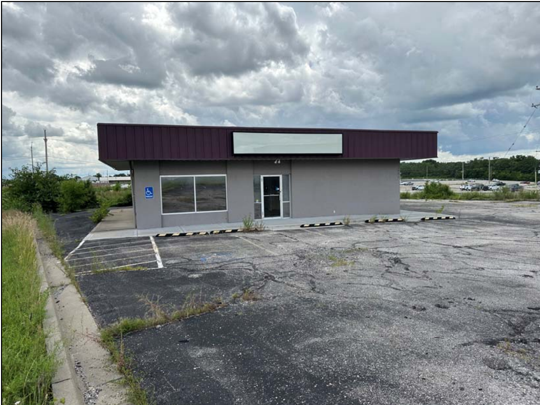
1031 SW Jefferson St – deterioration of parking pavement
