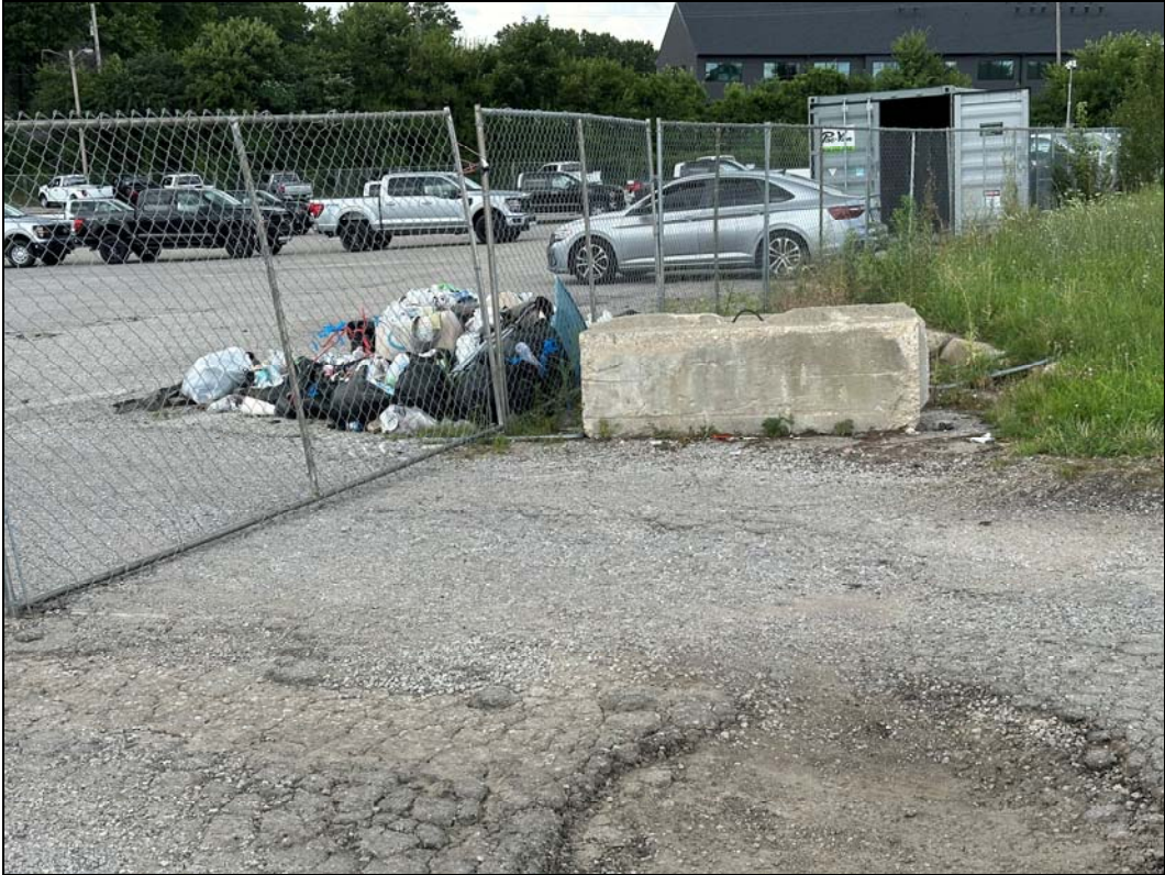
101 Oldham Pkwy – trash/debris; deterioration of pavement; overgrown vegetation
