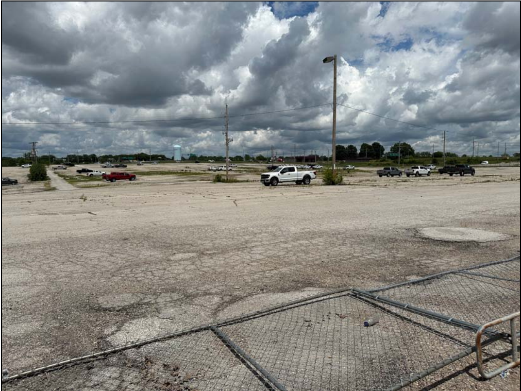
101 SW Oldham Pkwy – deterioration of pavement; overgrown vegetation; failure of finishes
