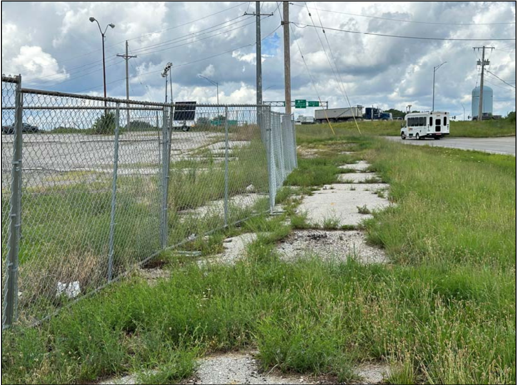
101 SW Oldham Pkwy – deterioration of pavement, fence; overgrown vegetation
