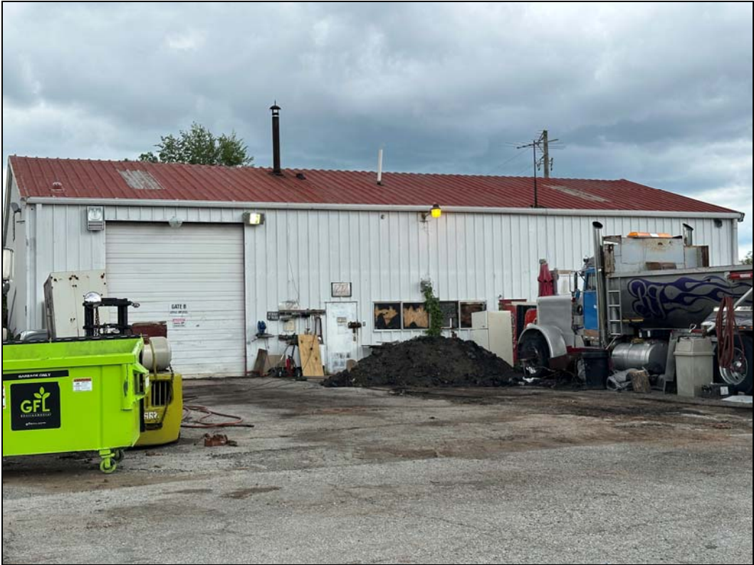
1212 SW Market St – failure of finishes; deterioration of windows, doors
