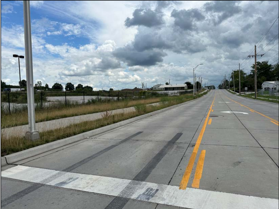
1035 SW Jefferson St – overgrown vegetation
