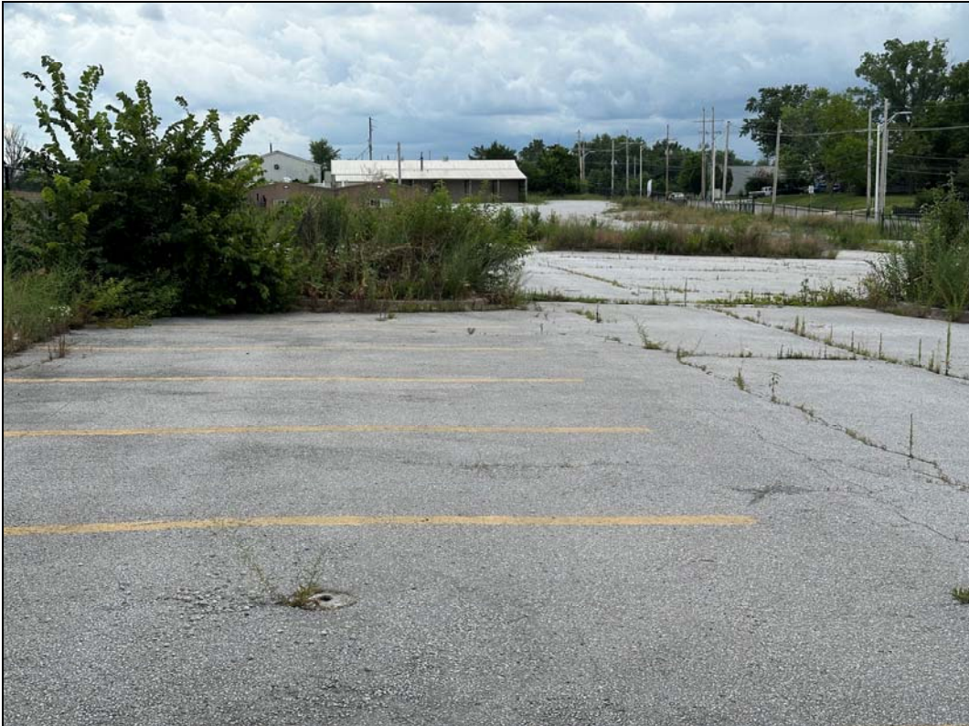
1035 SW Jefferson St – deterioration of parking lot; overgrown vegetation
