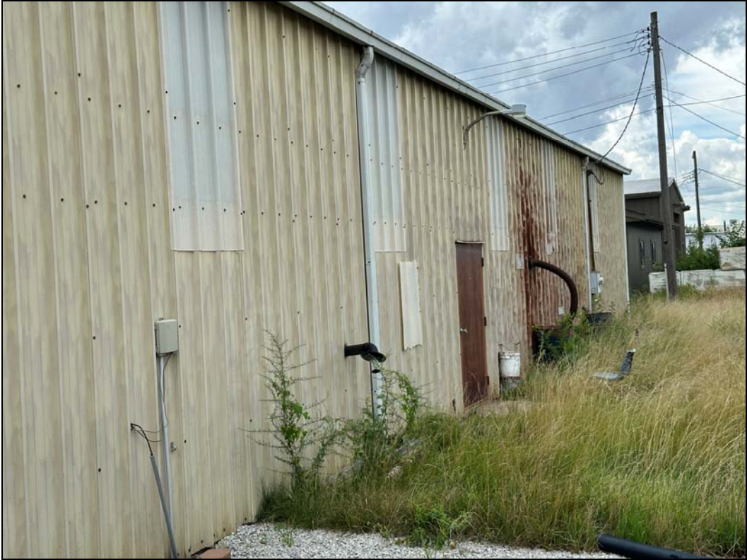
1313 SW Jefferson St – failure of finishes; deterioration of door; overgrown vegetation
