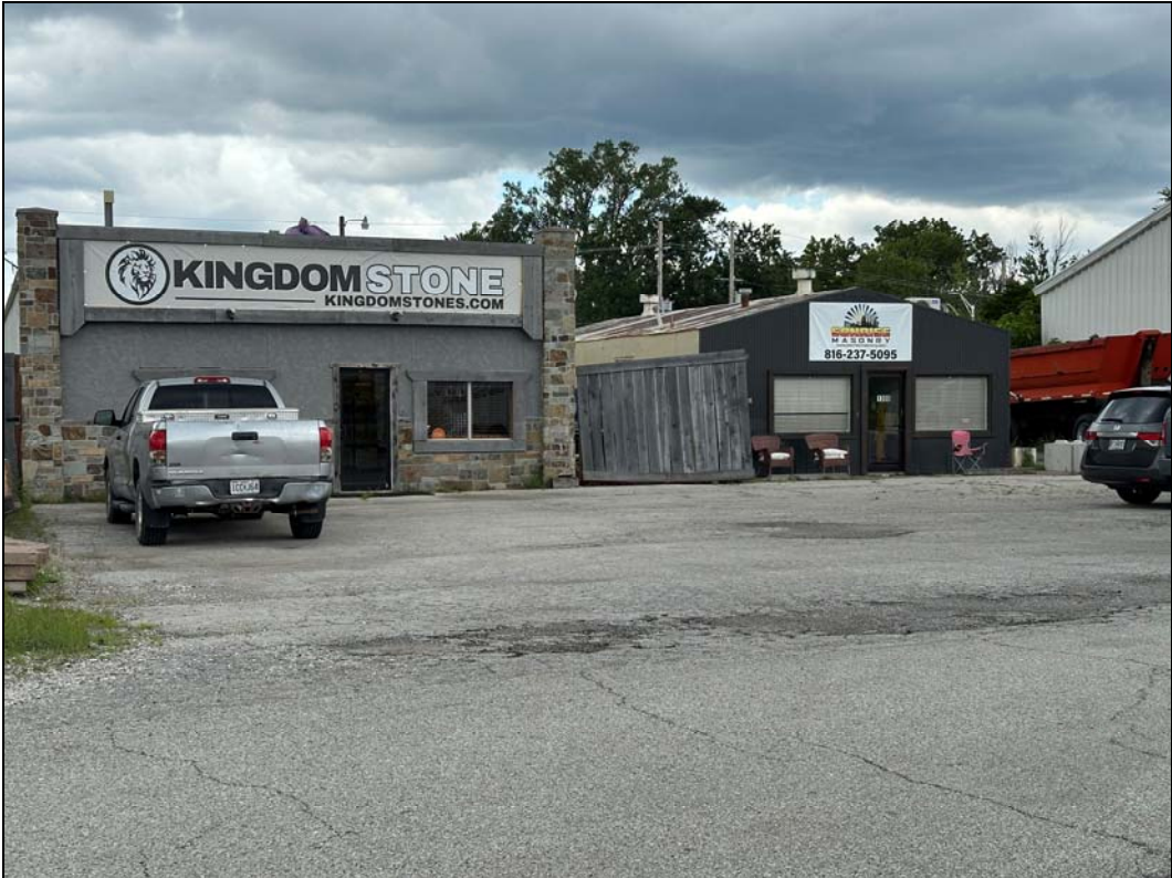
1300-1302 Market St – deterioration of pavement
