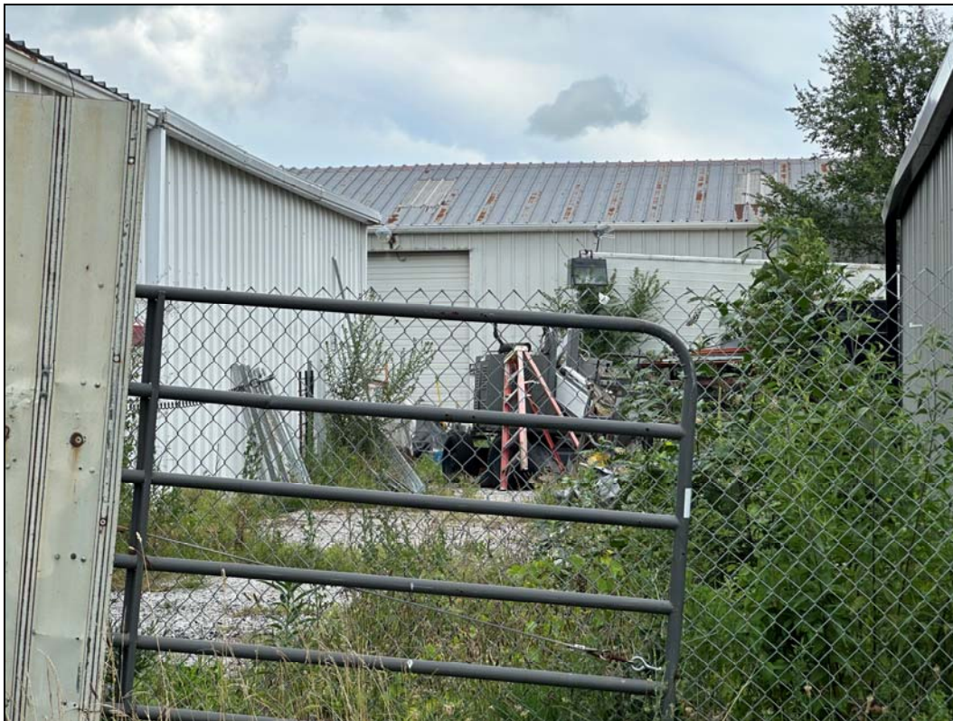
1212 SW Market St – failure of finishes (roof)
