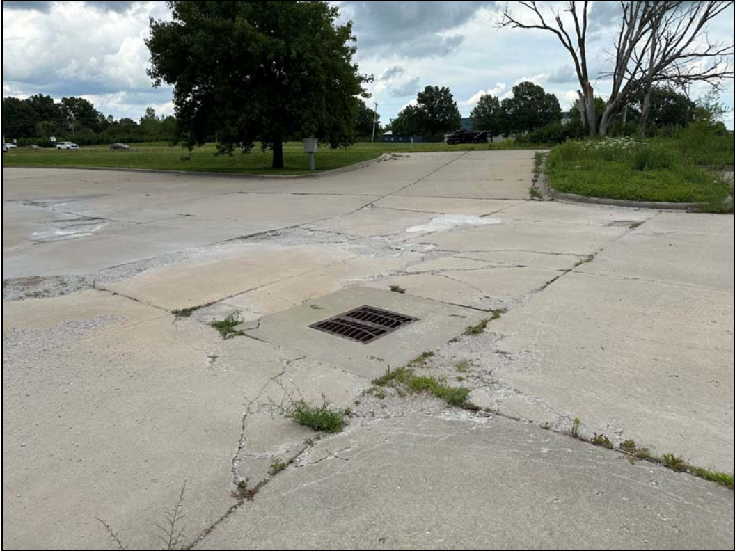
1306 SW Market St – deterioration of pavement; overgrown vegetation
