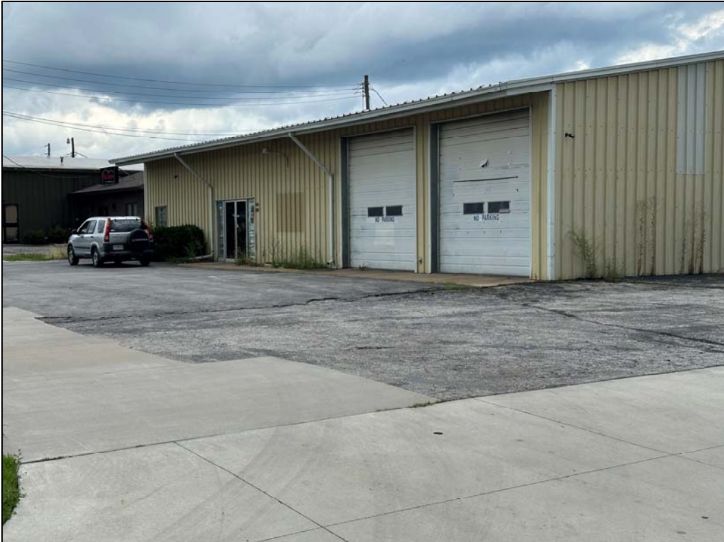
1313 SW Jefferson St – deterioration of doors; failure of finishes; deterioration of pavement
