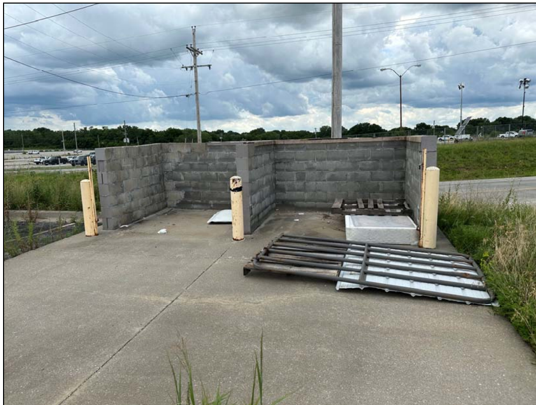
1031 SW Jefferson St – trash/debris; deterioration of trash enclosure
