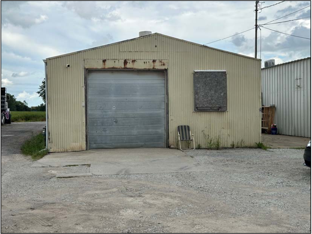
1300 SW Market St – deterioration of roof, windows, door; failure of finishes
