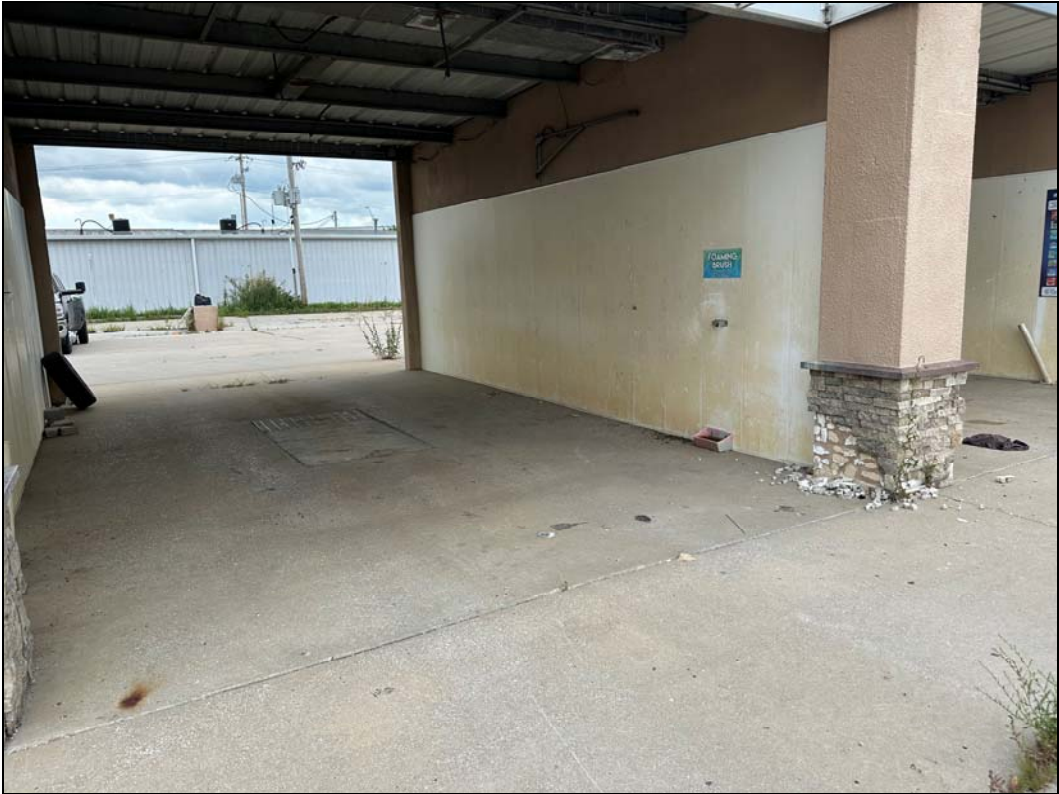
1310 SW Market St – damaged masonry veneer, equipment; trash/debris
