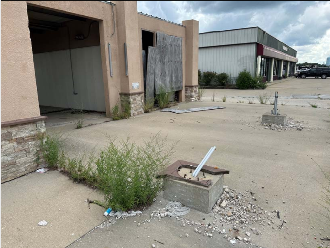
1310 SW Market St – deterioration of doors, masonry veneer, equipment
