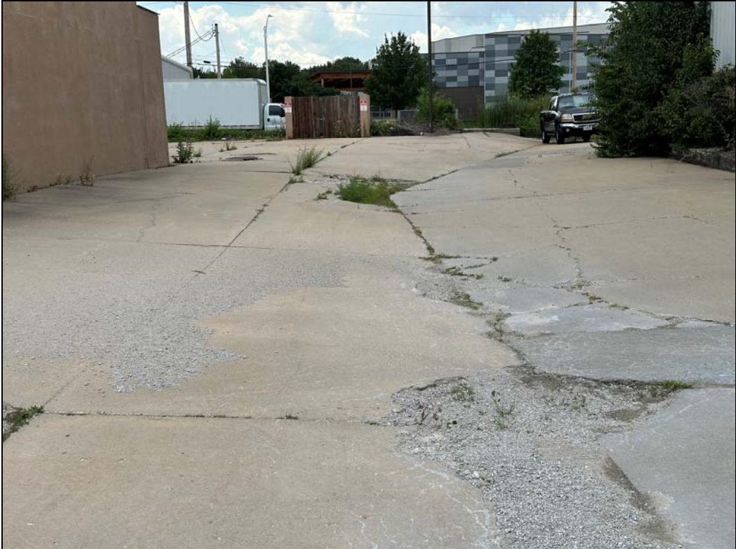
1306 SW Market St – deterioration of pavement
