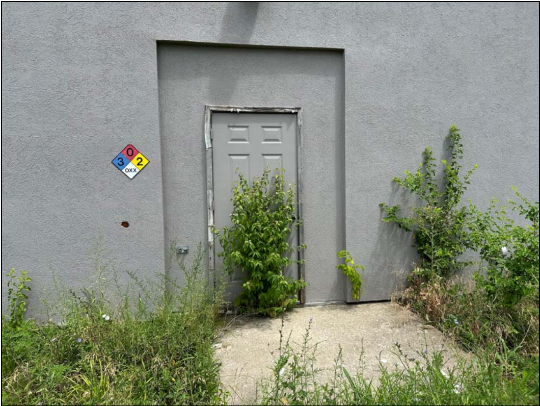
1025 SW Jefferson St – deterioration of door; overgrown vegetation
