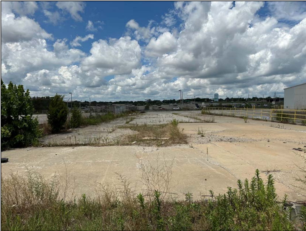
1204 SW Jefferson St – deterioration of pavement; overgrown vegetation
