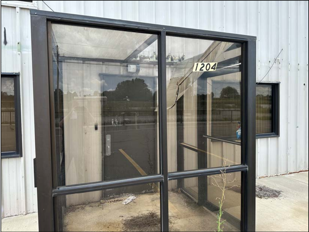
1204 SW Jefferson St – deterioration of entrance canopy; failure of finishes
