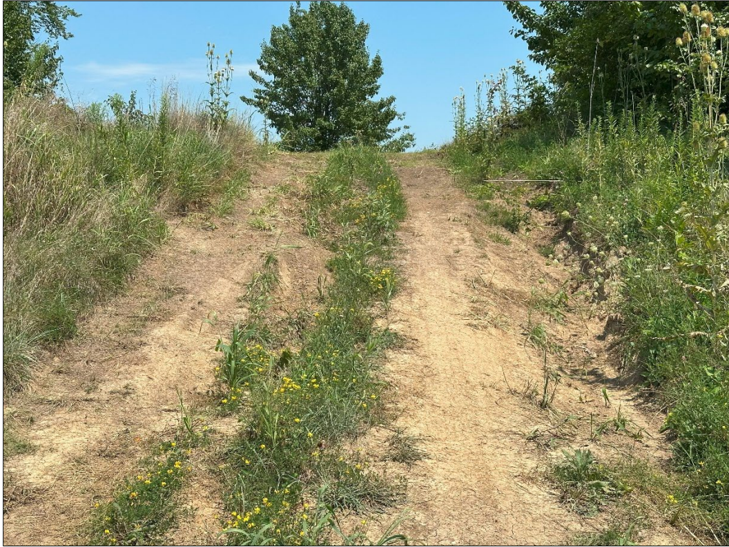
1001 S. M-291 – looking east – open access; deterioration of drive
