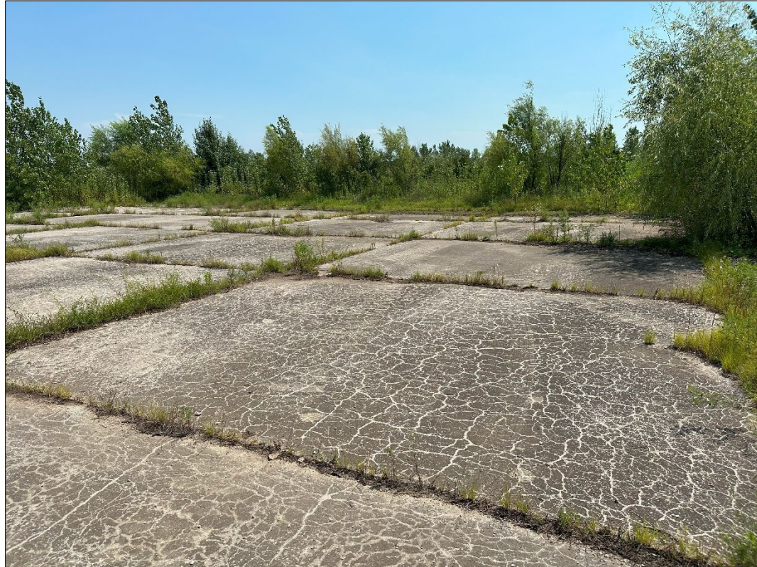
1001 S. M-291 – looking southeast – deterioration of pavement; overgrown vegetation
