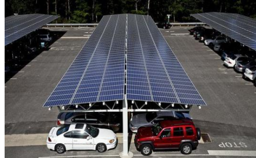
Fig.6.480.C-1: Accessory solar arrays in a parking lot
