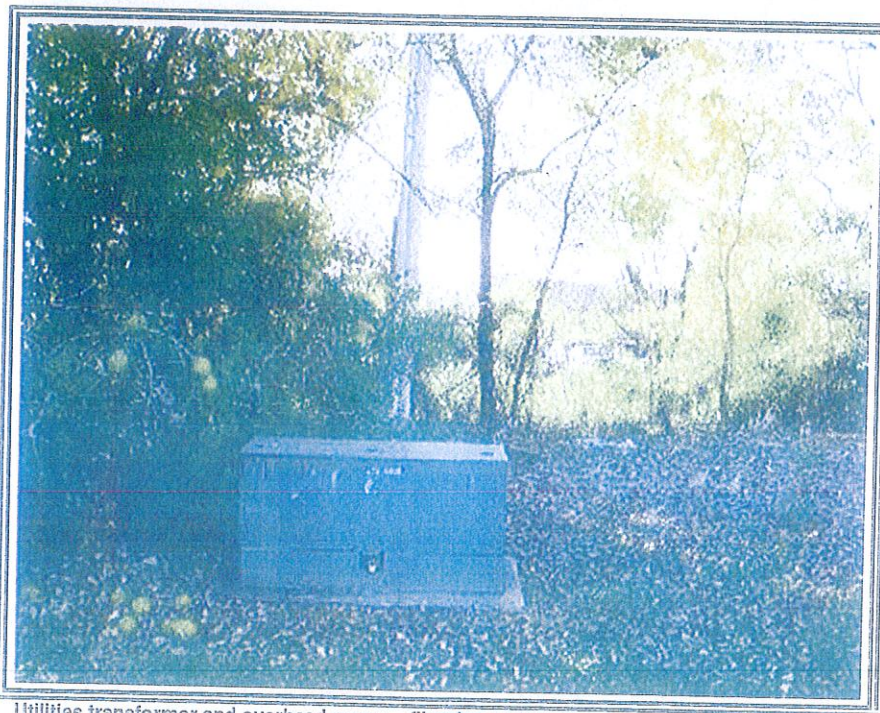
Utilities transformer and overhead power – fiber located western edge of parcel
