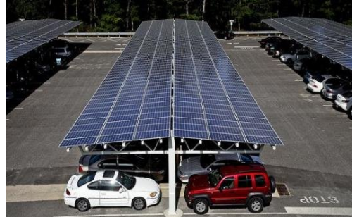
Fig.6.480.C-1: Accessory solar arrays in a parking lot
