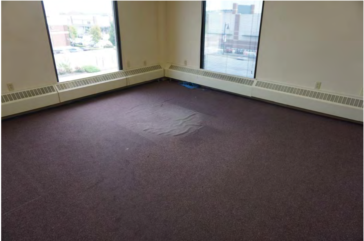
Representative interior view of vacated space in need of updating
