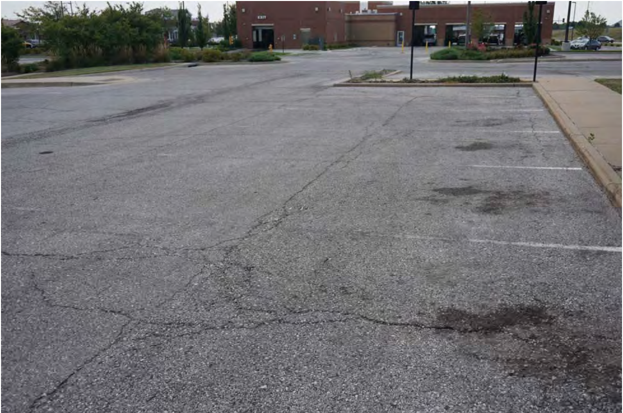
Representative view of the parking area with signs for deterioration and neglect
