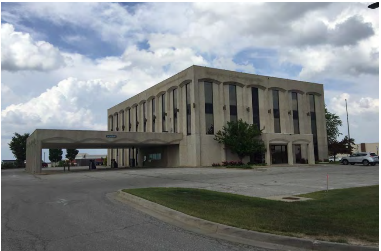
Representative exterior view of the Study Area with signs for deterioration and aging
