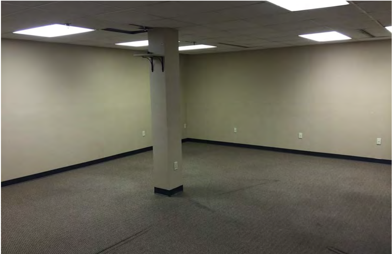
Representative interior view of vacated space with aging finish and deterioration
