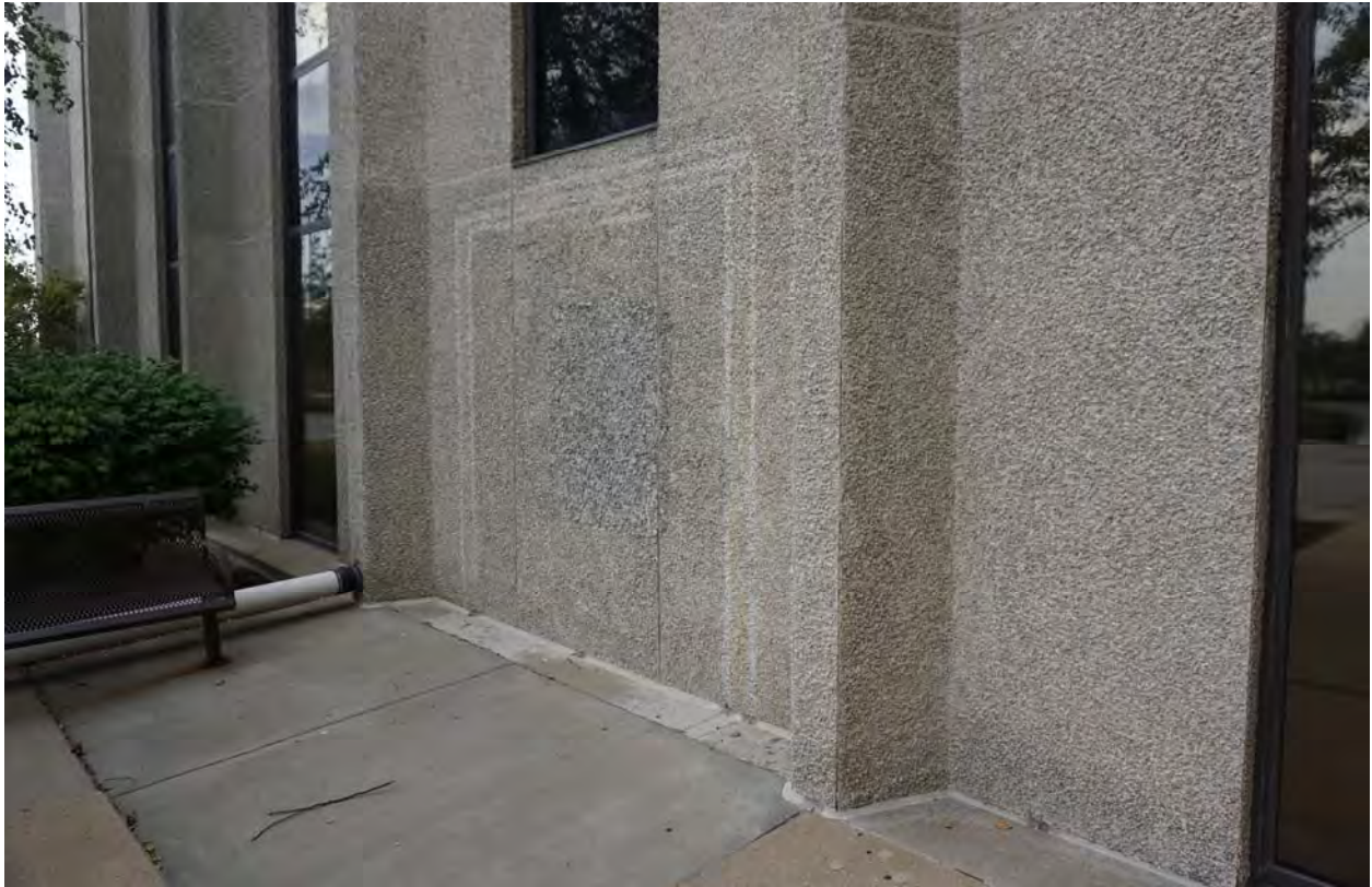
View of exterior façade with deterioration
