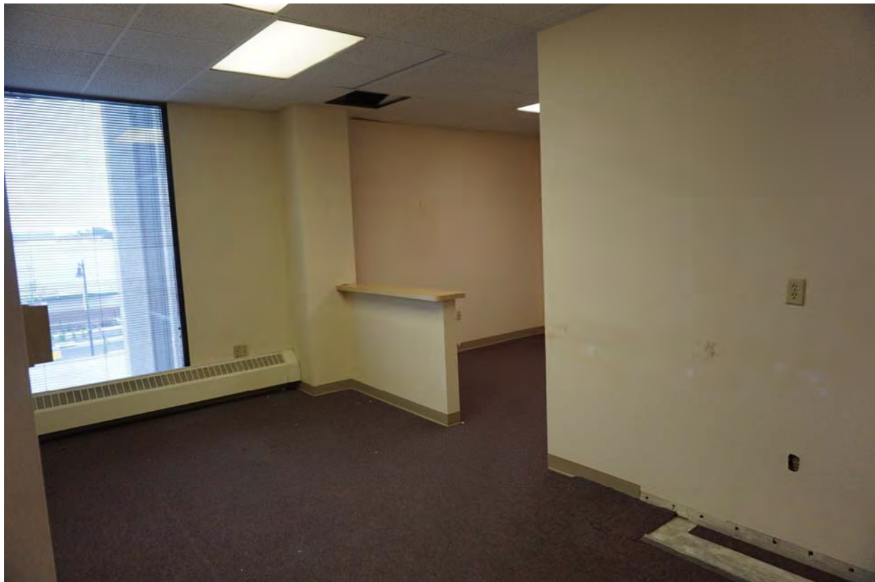
Aging interior improvements that will need to be updated before future occupancy can occur
