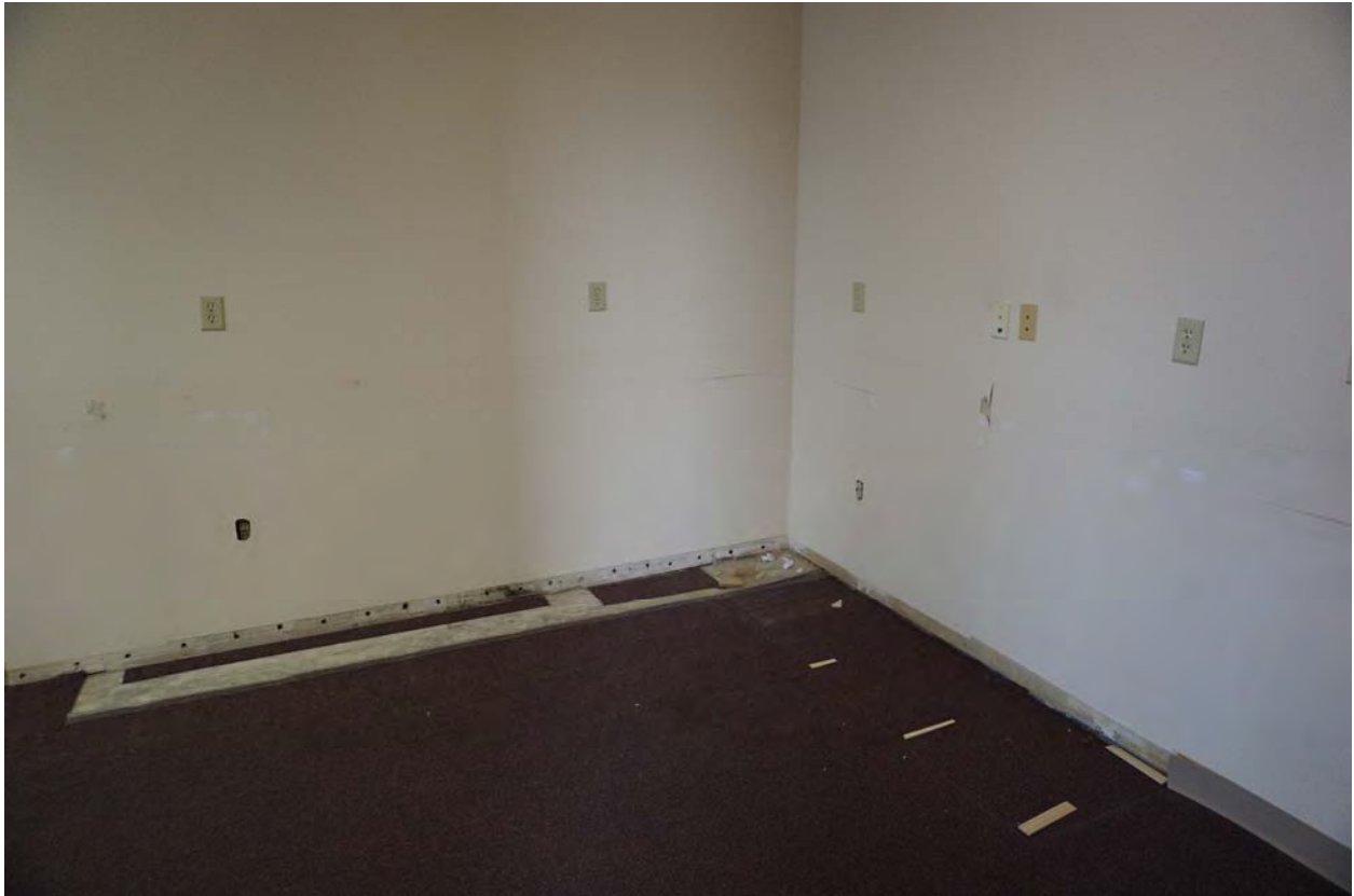
Representative interior view of in need of updating
