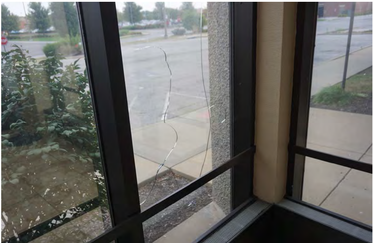
View of broken glass in the interior lobby
