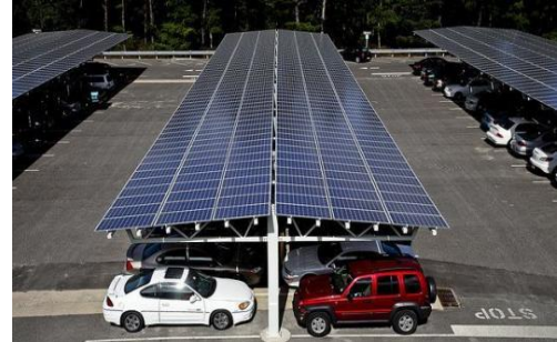
Fig.6.480.C-1: Accessory solar arrays in a parking lot
