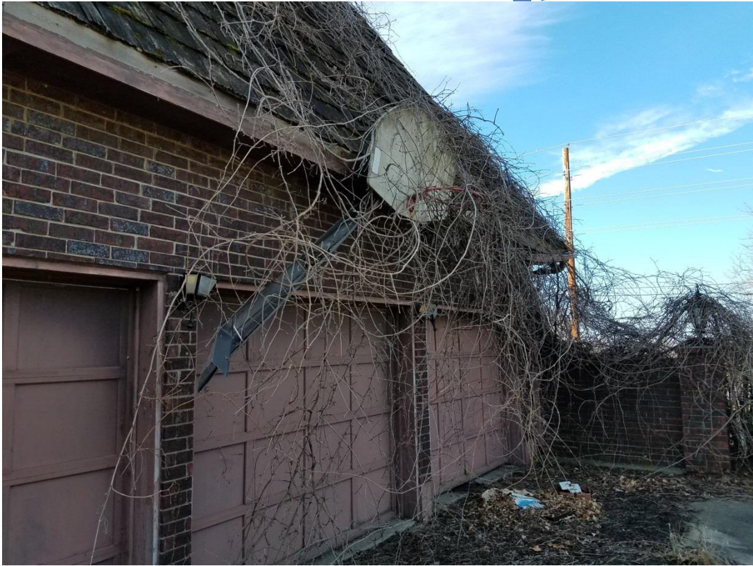
Photo 9 – View of overgrown ivy/vine landscaping at the garage location.
