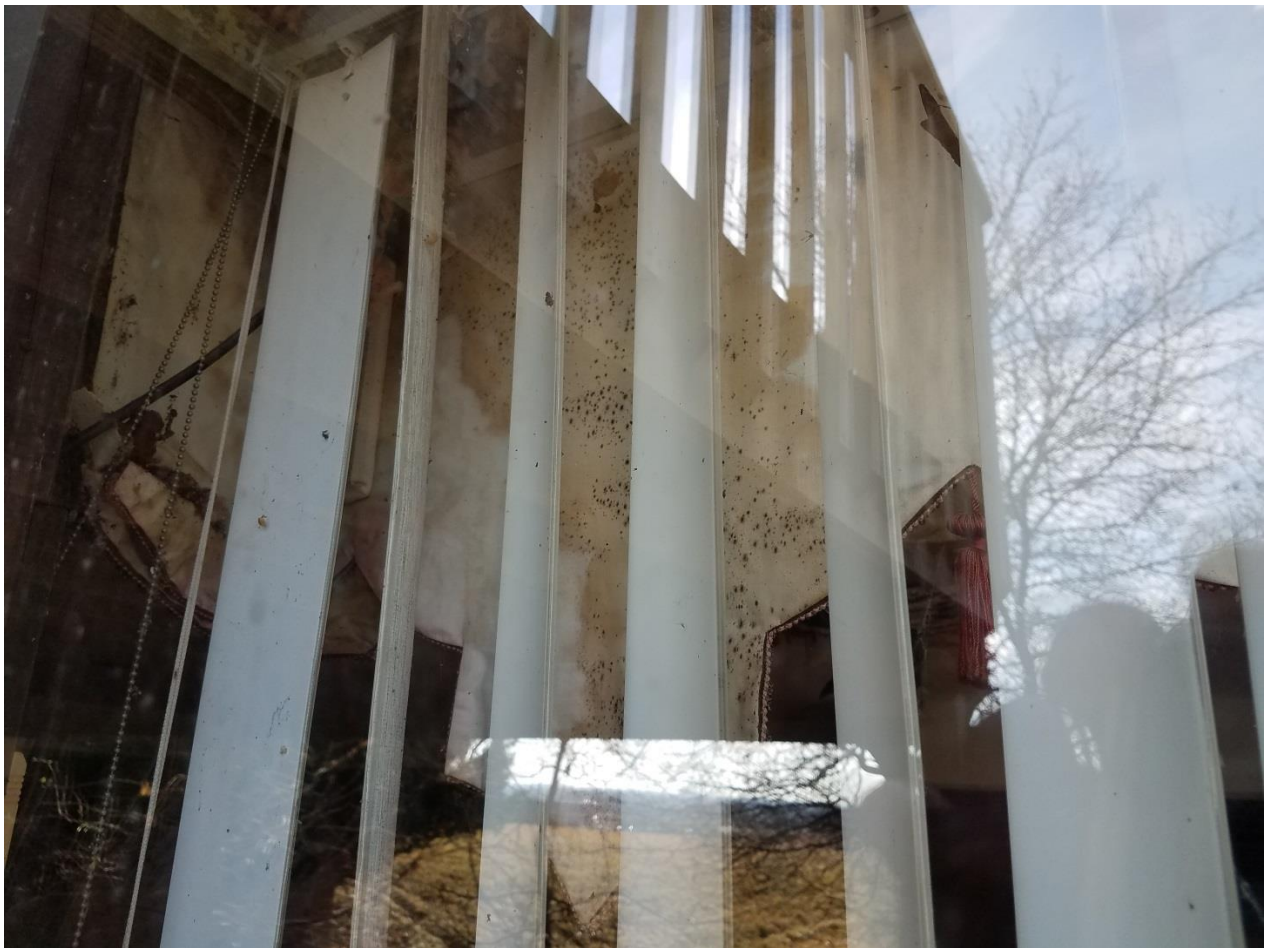
Photo 11– View of suspect black mold (note black spots on interior curtains) on interior surfaces within the basement of 225 SW High Dr.
