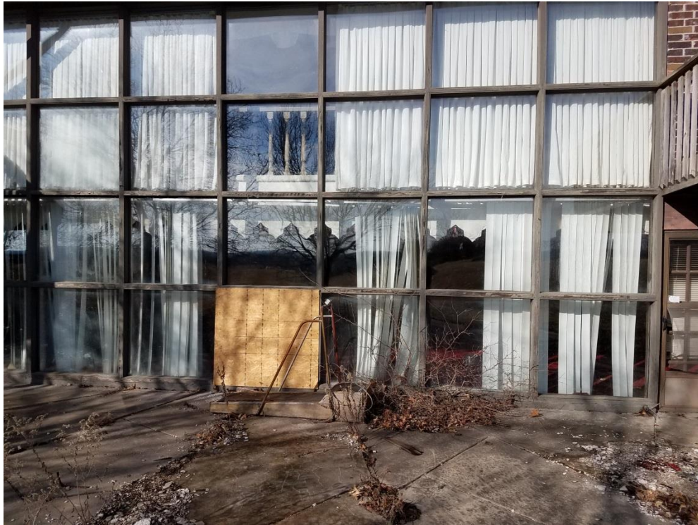
Photo 8 - View of the east side of vacant residence. Note boarded window.
