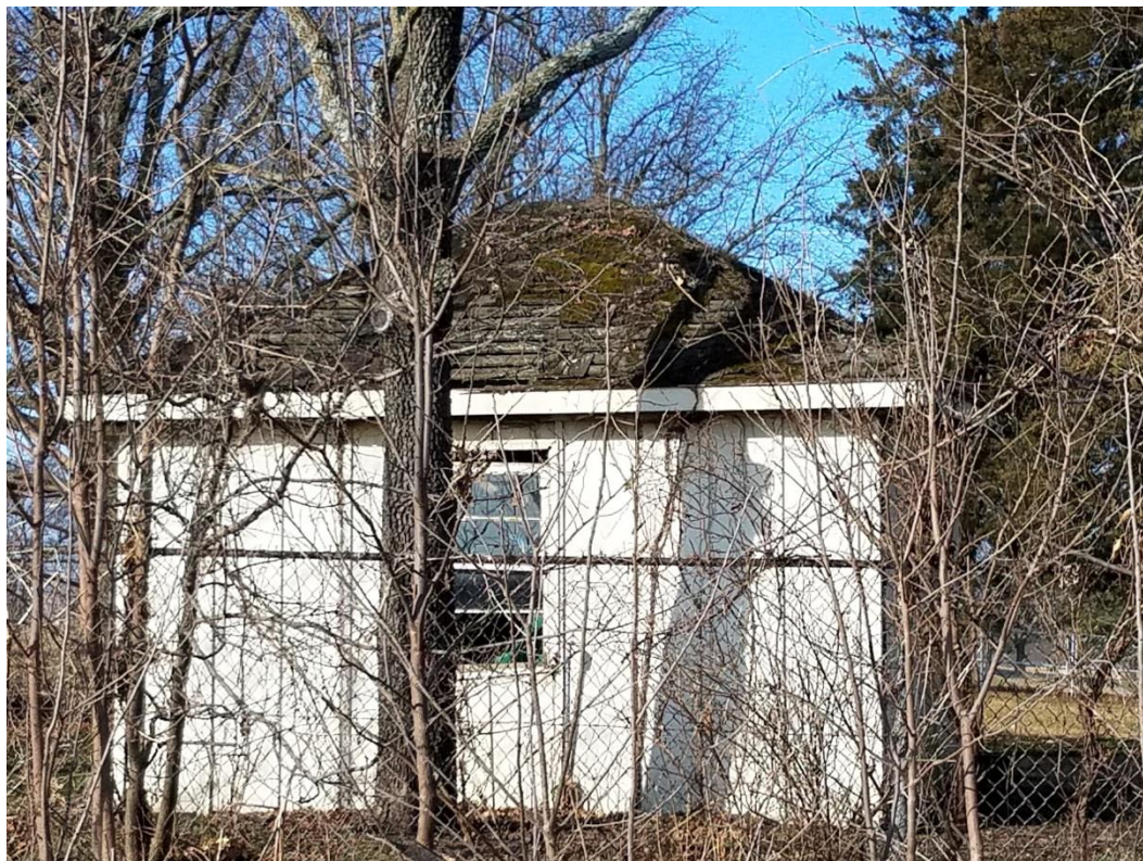
Photo 23 – View of accessory structure (11401 SW View High Dr.). Note severely deteriorated roof.
