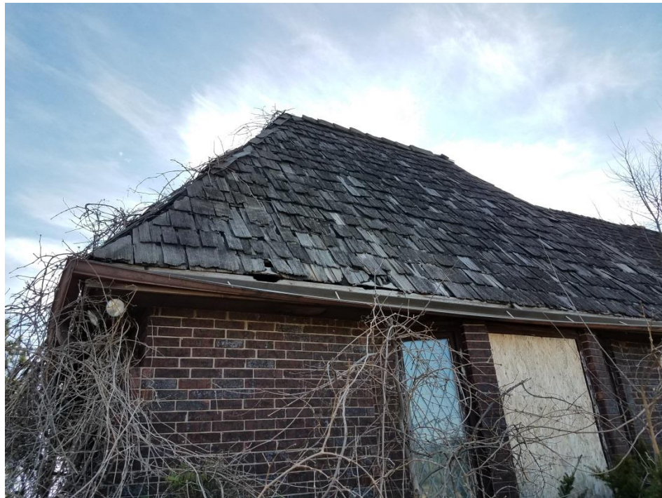
Photo 7 – Roof and structure deterioration. Note boarded, broken window.
