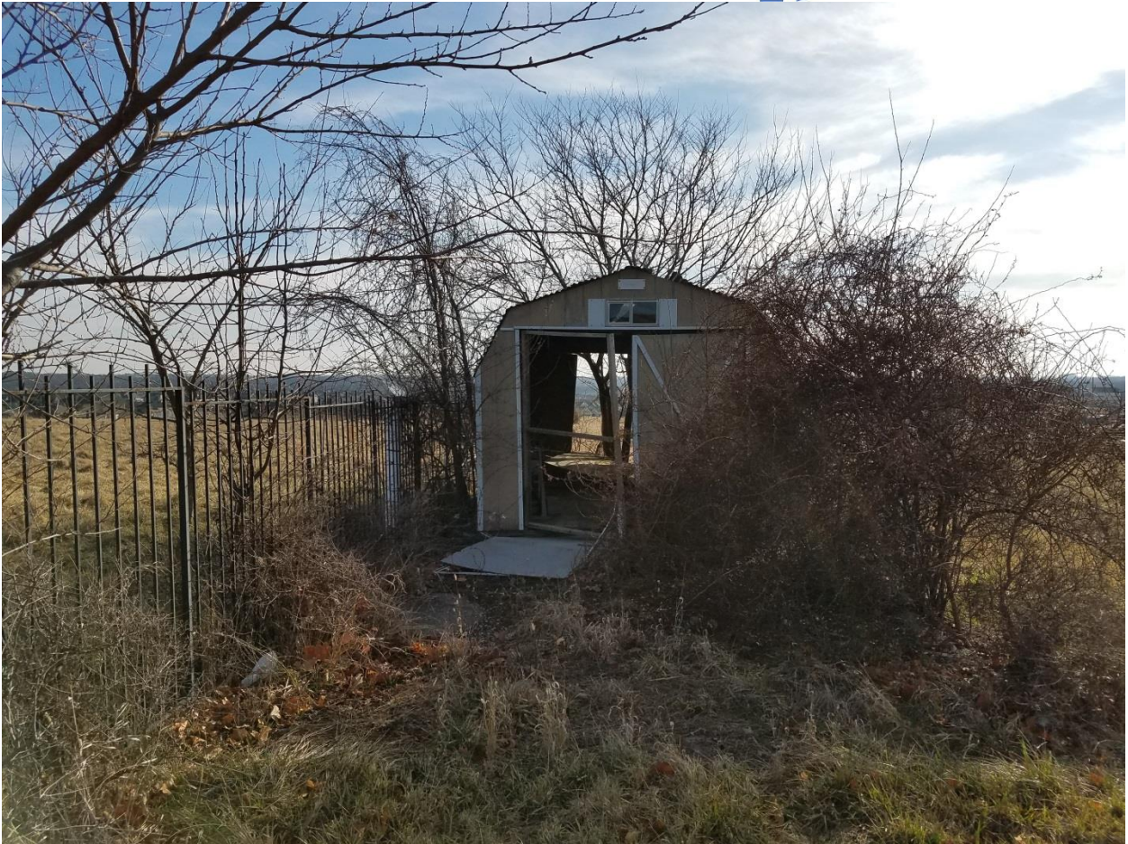
Figure 24 – Severely deteriorated accessory structure located on Parcel #1.
