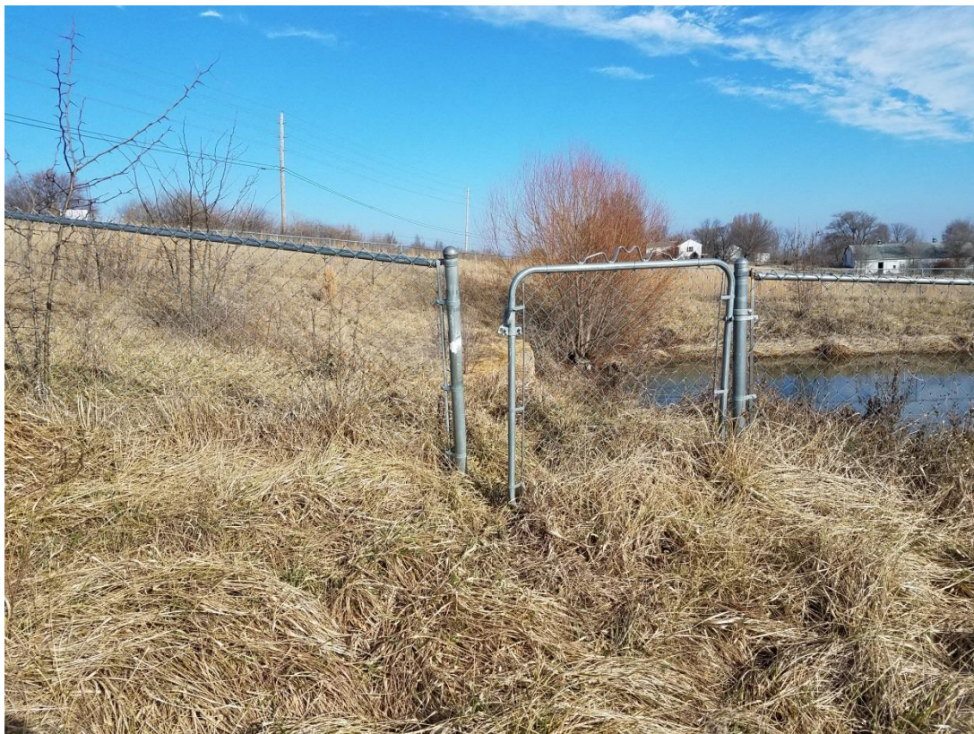
Photo 21 – View of gate access to septic pond. Gate is stuck open due to overgrown vegetation.
