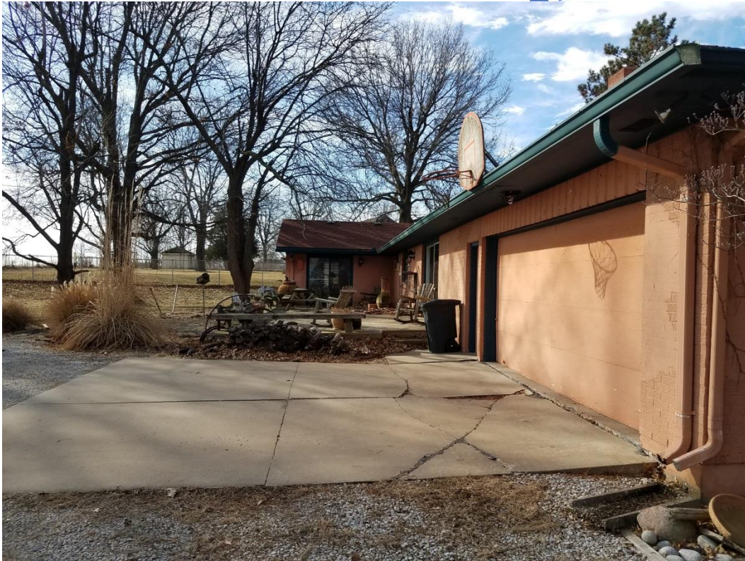
Photo 22 – View of the rear garage at 11303 SW View High Drive. Note severe cracking on driveway, a possible indication of possible foundation settling.
