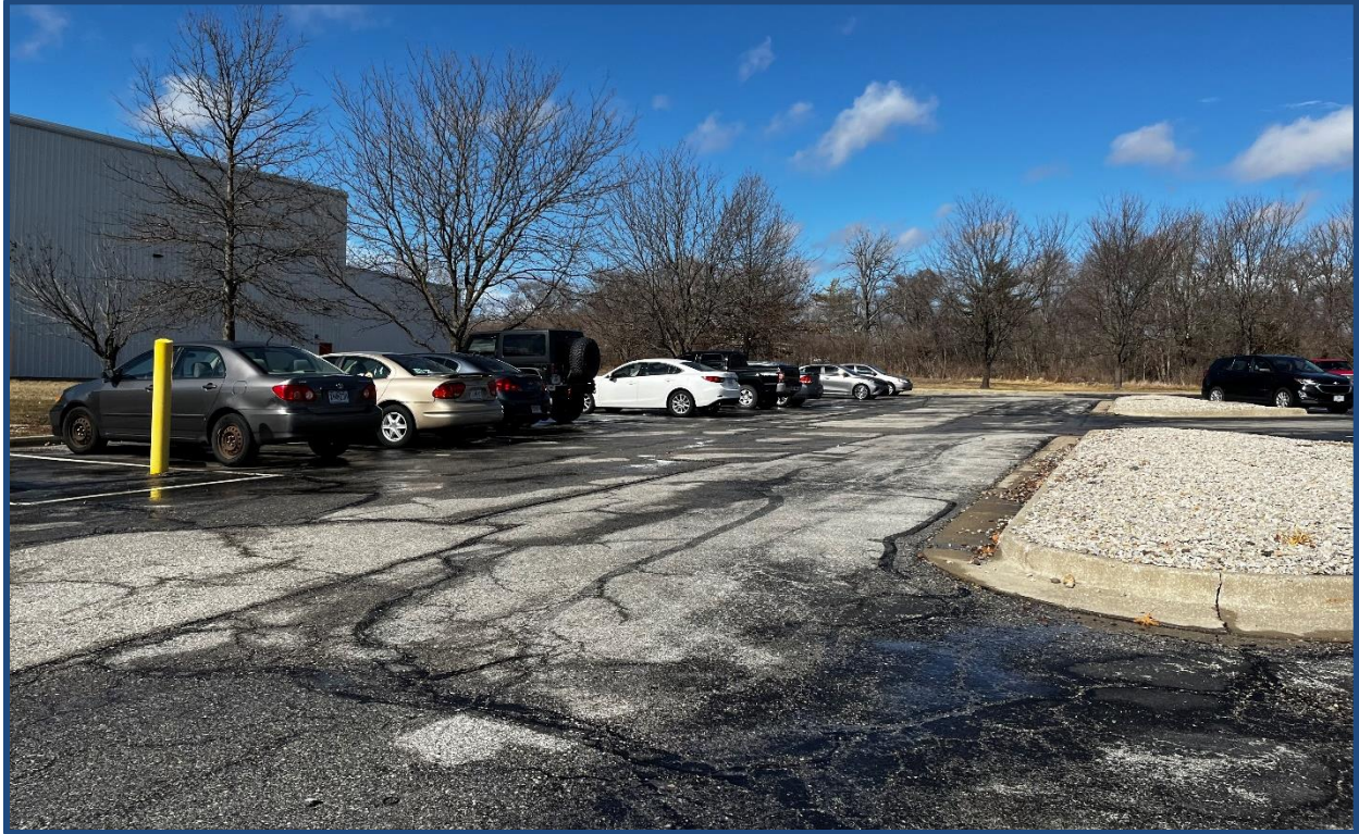
Representative site view of the existing facility with parking deterioration
