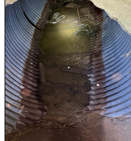
Corrugated Metal Pipe Deterioration
