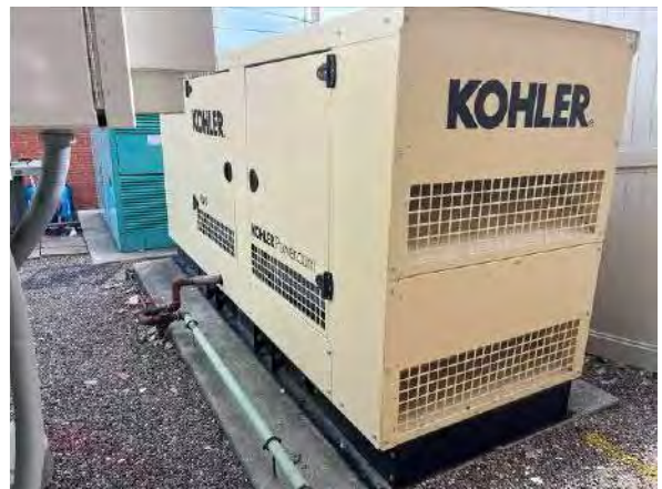
Photo #12 View of natural gas emergency generator
