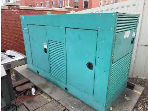
Photo #13 View of natural gas emergency generator
