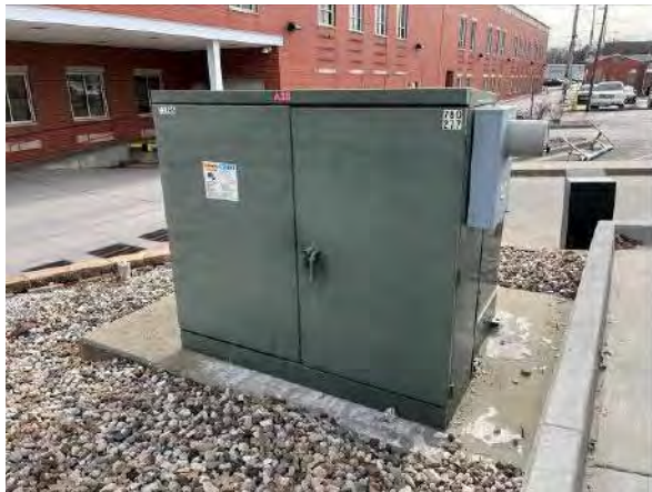
Photo #15 View of on-site pad-mounted transformer
