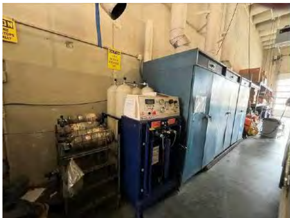
Photo #17 View of oxygen tank storage in Bay
