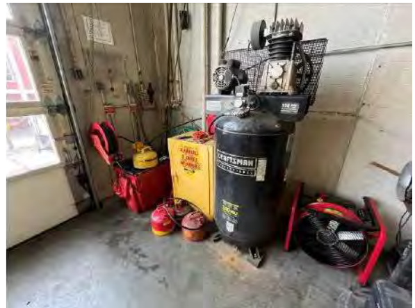
Photo #16 View of air compressor and four ~3-5 gallon gas/diesel cans
