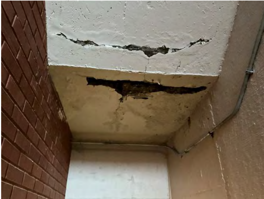
Figure 1: North exit stair concrete spall.
