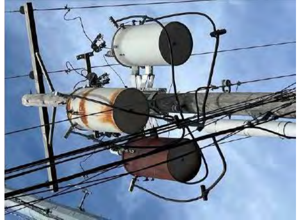
Photo #14 View of on-site pole-mounted transformers
