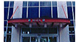
Canopy or Marquee Sign
