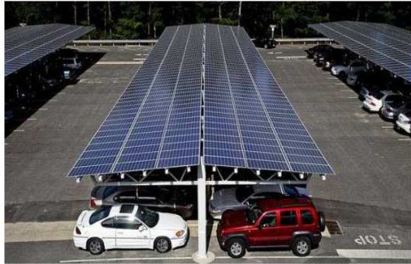
Figure 5.510.C-1: Accessory Solar Arrays in a Parking Lot
