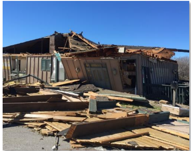
Photo 4: Damage from EF-0 Tornado (March 6, 2017)
