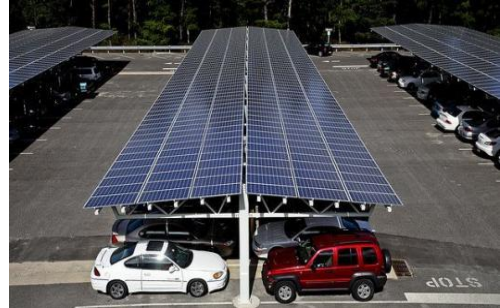
Fig.6.480.C-1: Accessory solar arrays in a parking lot
