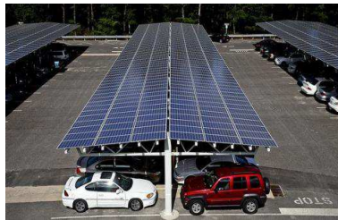
Fig.6.480.C-1: Accessory solar arrays in a parking lot
