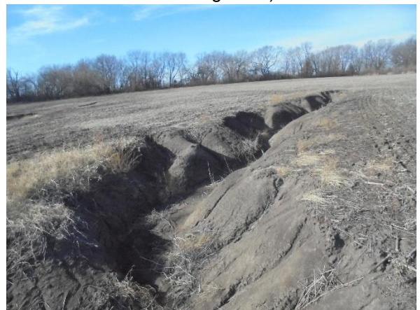
Photo #12 View of erosional feature on the central portion of the site.
