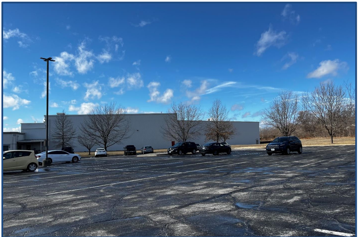
Representative site view of the existing facility with parking deterioration
